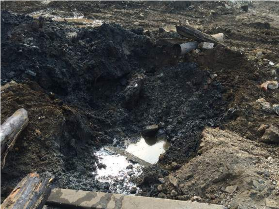
Photograph 16: View of the petroleum-impacted soil that was observed beneath UST-15.
