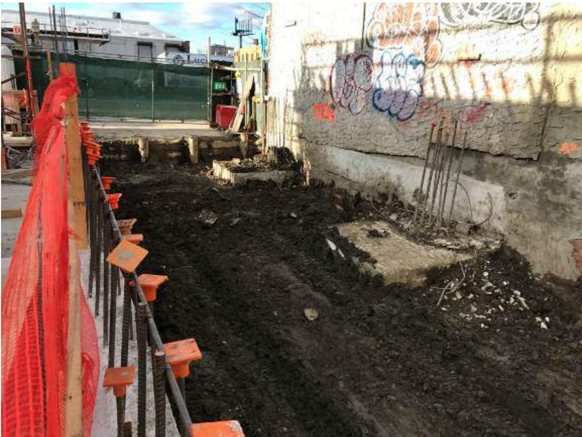
Photograph 122: Additional view of the southern portion of the ramp prior to stone import, facing west.
