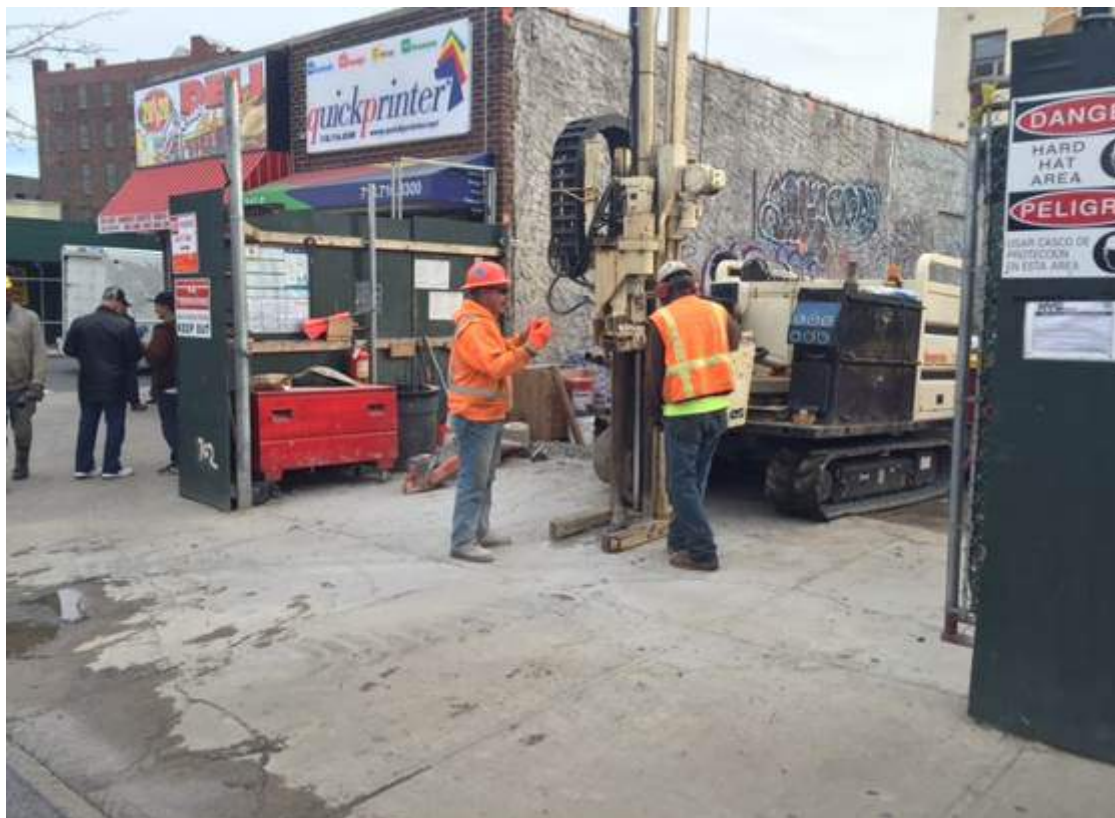
Photograph 52: View of AARCO installing the permanent monitoring well (SMW-1) in the East 138 th Street sidewalk, facing north.
