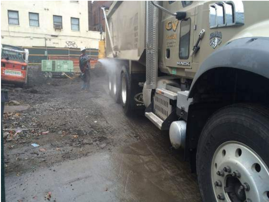
Photograph 45: View of the contractor applying water to the truck wheels prior to exiting the Site.
