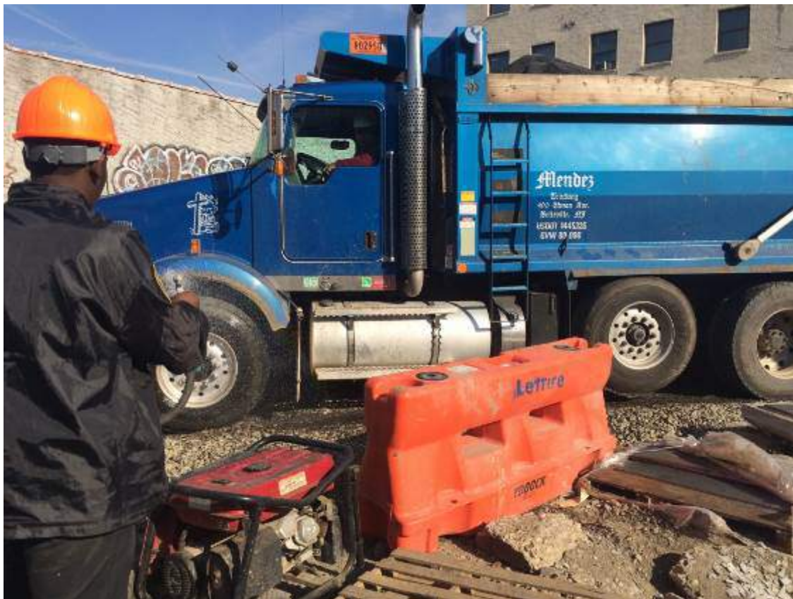
Photograph 39: View of the contractor applying water to the truck wheels prior to exiting the Site, facing north.
