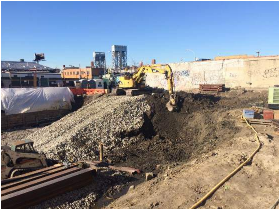
Photograph 46: View of the contractor excavating in the western portion of the Site, facing west.
