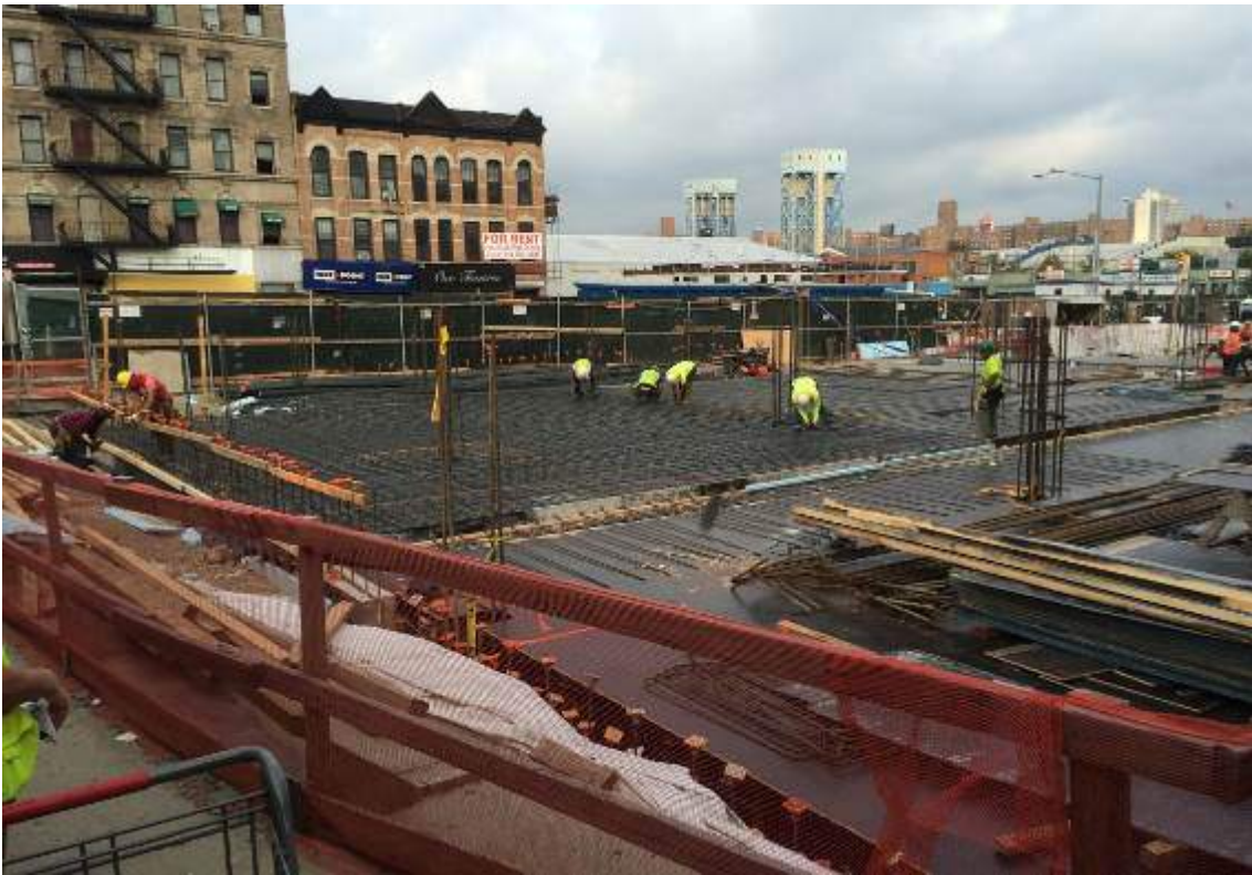
Photograph 83: View of the contractor installing the framing and rebar for the first floor in the southeastern portion of the Site, facing northwest.
