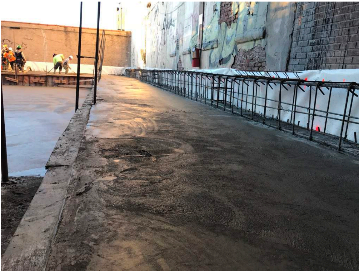
Photograph 135: View of the installed concrete along the northern boundary of the Site, facing northwest.
