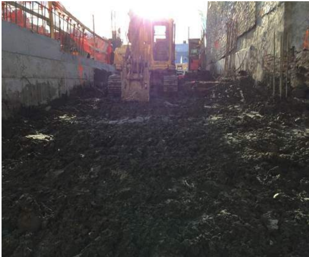
Photograph 121: View of the entrance ramp along the western boundary of the site, facing southwest.
