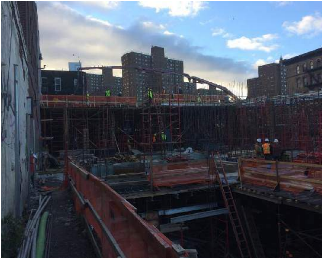
Photograph 105: View of the contractor working on the superstructure in the central and eastern portions of the site, facing southeast.
