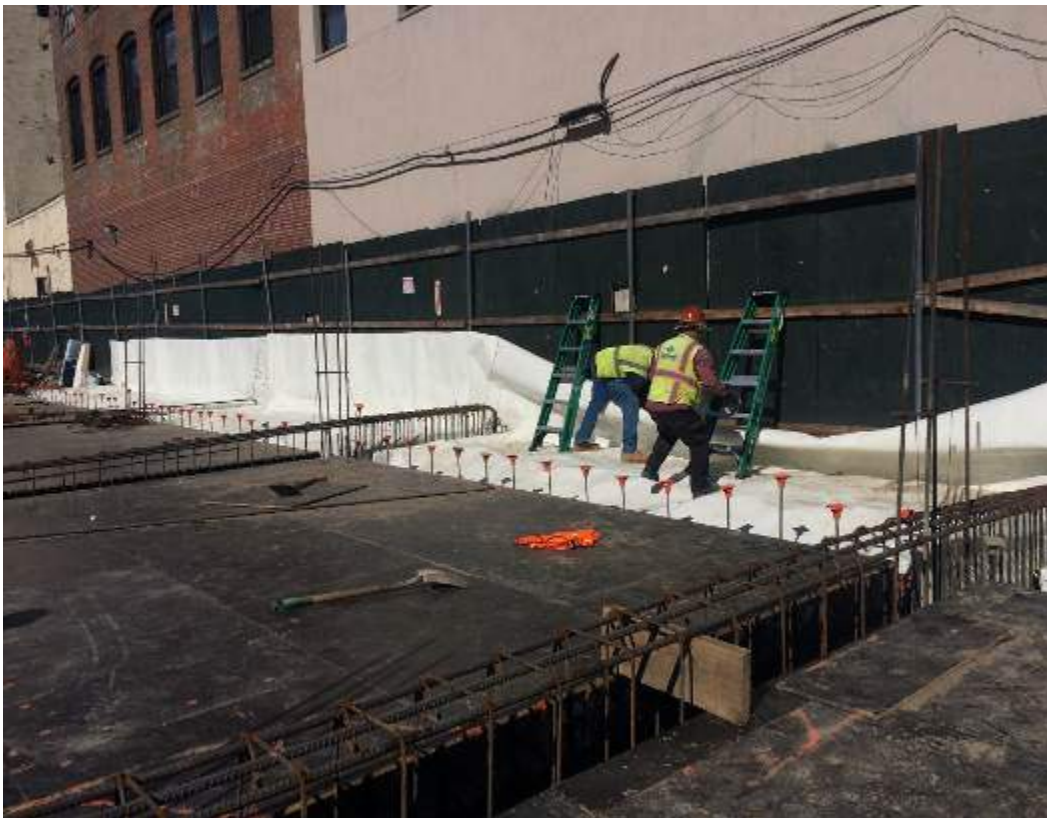
Photograph 90: View of the installed waterproofing membrane along the northern boundary of the Site, facing north.
