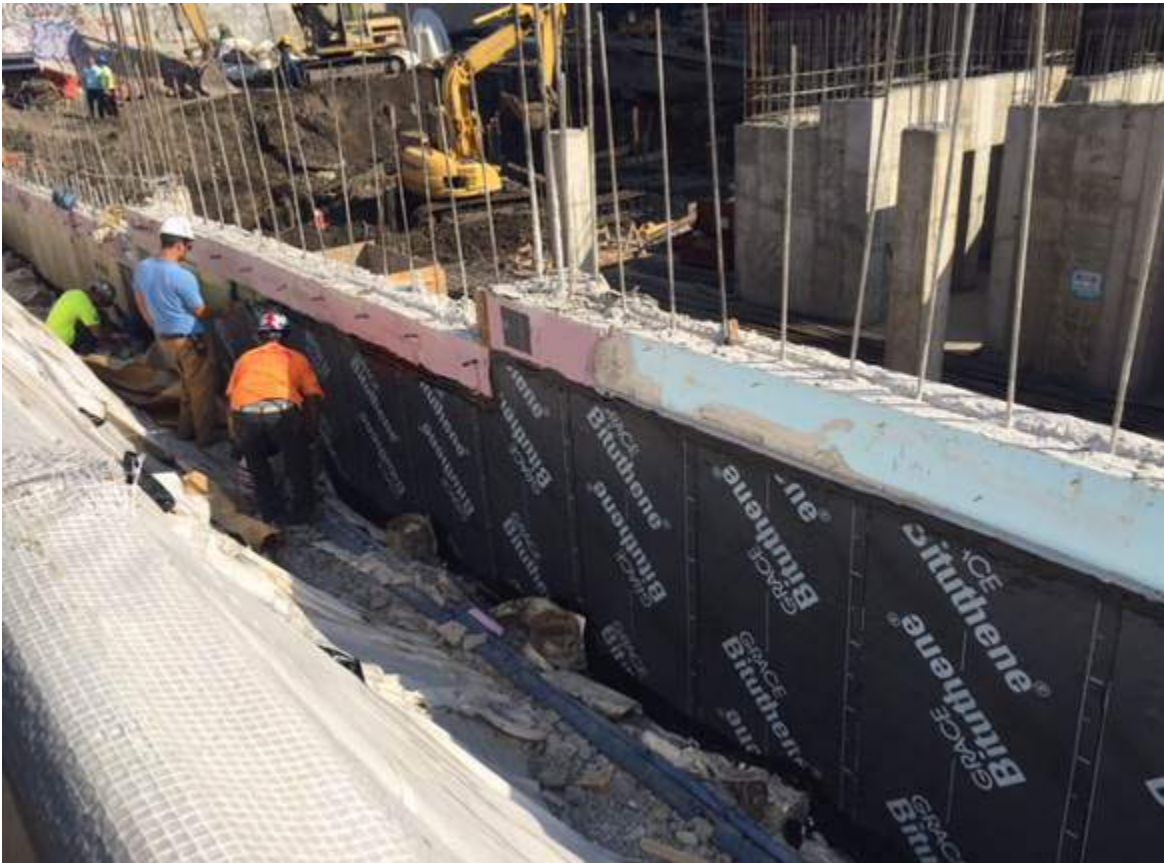
Photograph 77: View of the contractor installing the waterproofing membrane along the exterior portion of the southern boundary of the Site.
