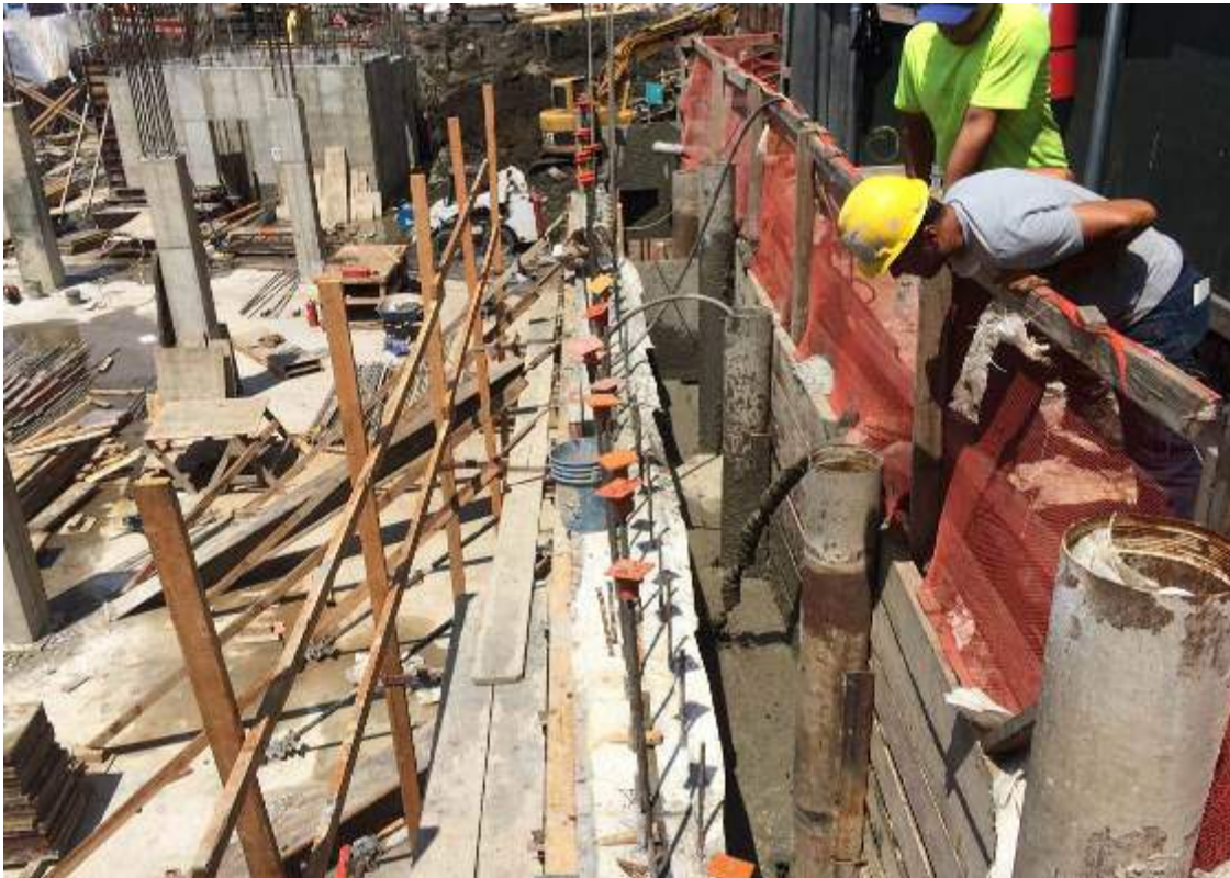
Photograph 74: View of the contractor pouring concrete between the foundation sidewall and lagging installation along the northeast boundary of the Site, facing northwest.
