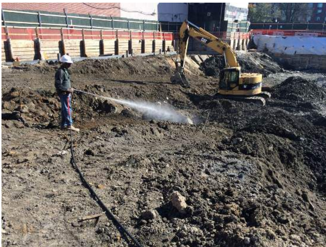
Photograph 40: View of the contractor using the LANDA 3500 PSI Power Washer to apply the BioSolve ® Pinkwater vapor suppressant to the petroleum-impacted soil.
