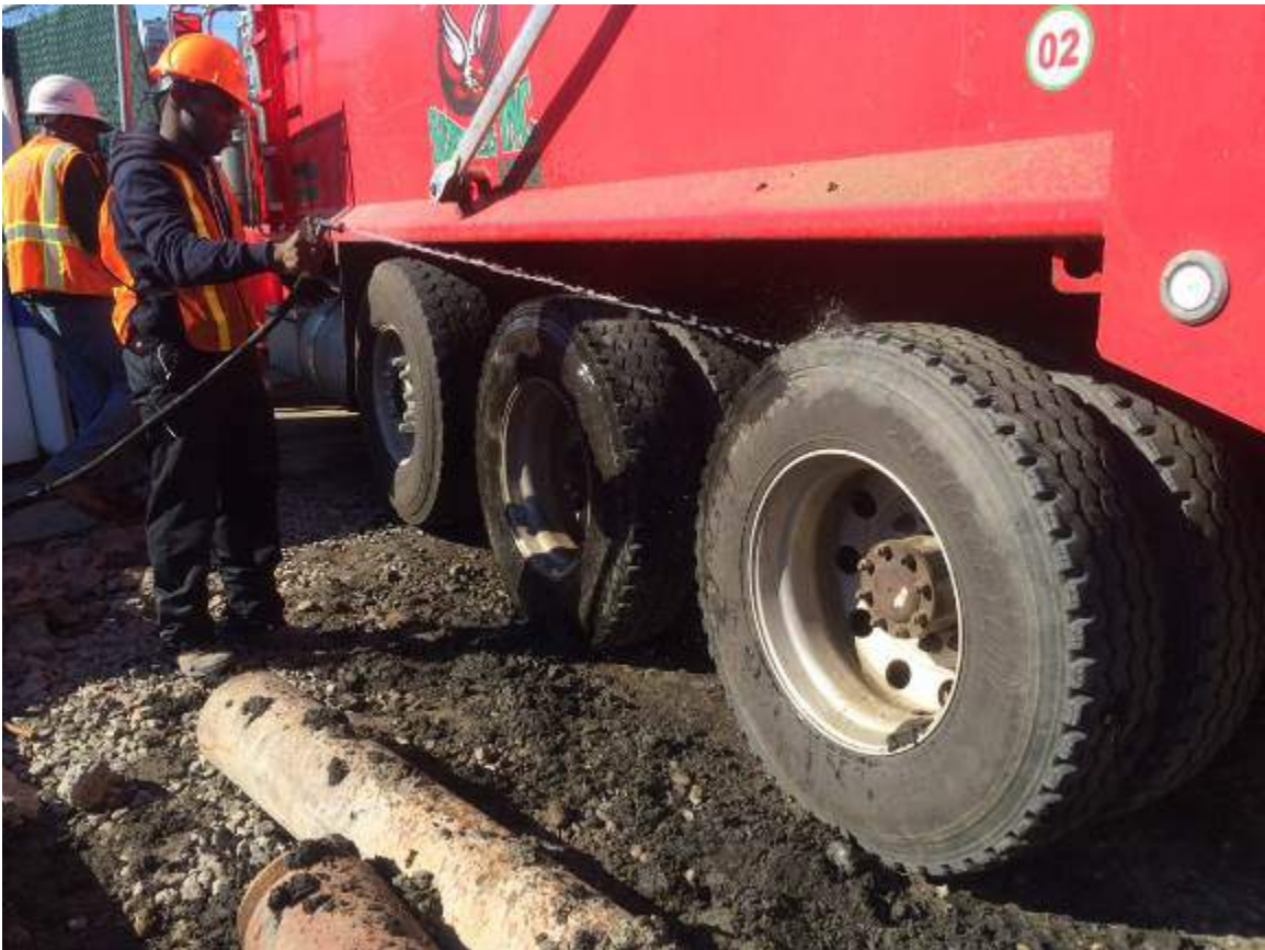
Photograph 41: View of the contractor cleaning the trucks with water prior to exiting the Site.
