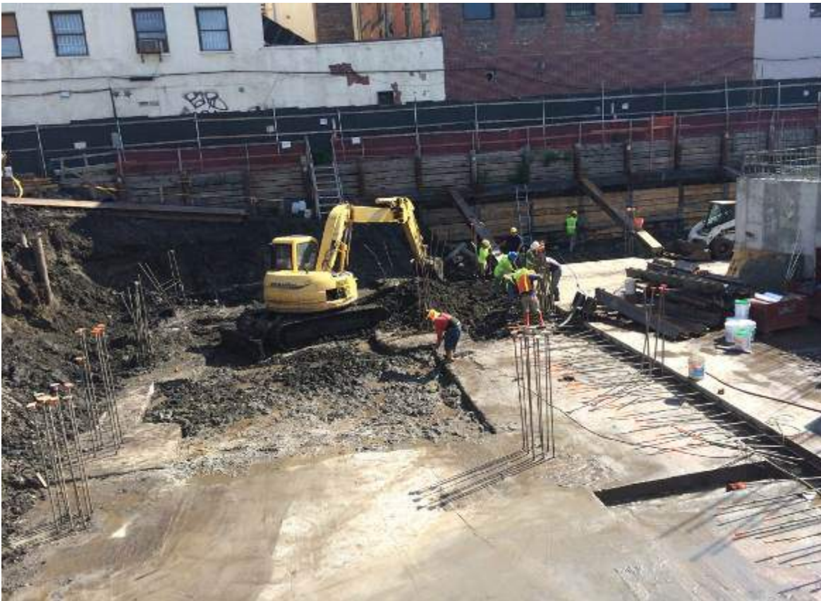
Photograph 78: View of the contractor excavating soil in the western portion of the Site, facing north.
