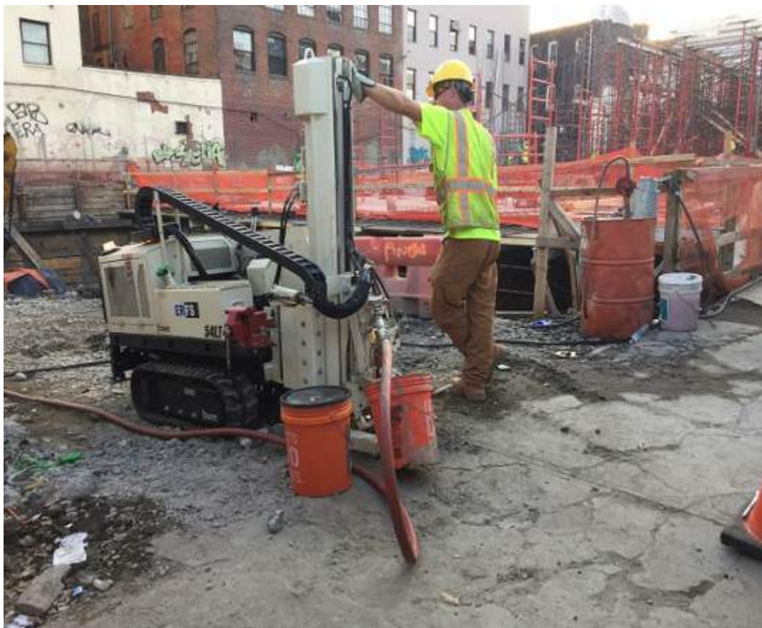
Photograph 96: View of ERFS advancing the temporary direct-push injection point TP-4, facing east.
