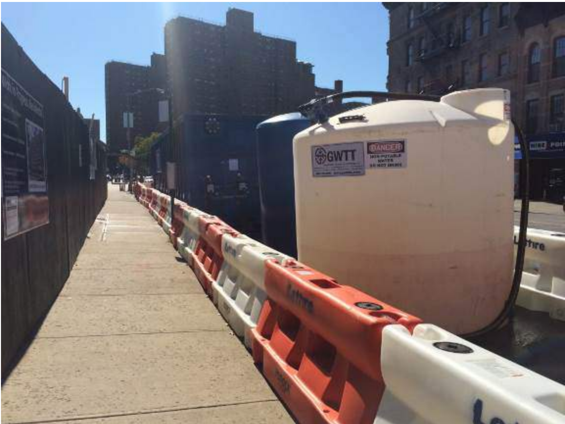
Photograph 24: View of the dewatering treatment system located along E. 138 th Street.
