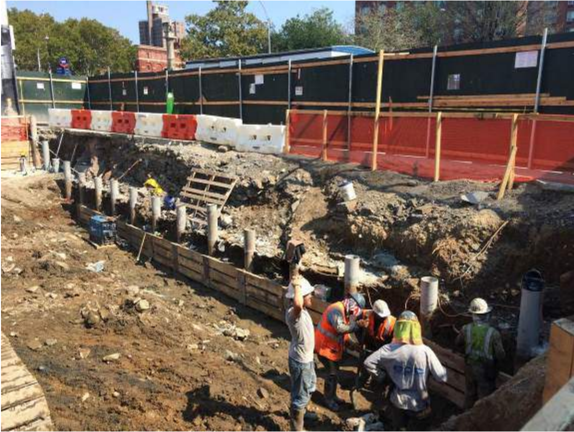
Photograph 27: View of the lagging installation progression along the eastern boundary of the Site, facing east.
