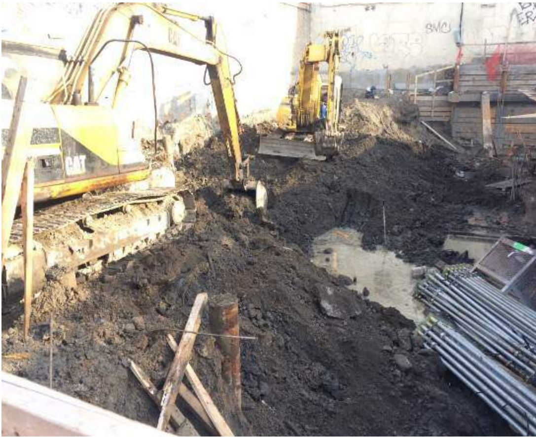
Photograph 107: View of the contractor excavating for the ramp along the western boundary of the Site, facing north.
