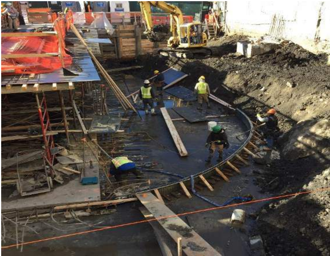
Photograph 117: View of the contractor preparing the western portion of the site for the Preprufe 300R waterproofing membrane installation, facing west.
