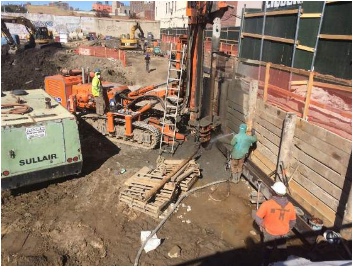
Photograph 35: View of the foundation pile installation along the northern boundary of the Site.
