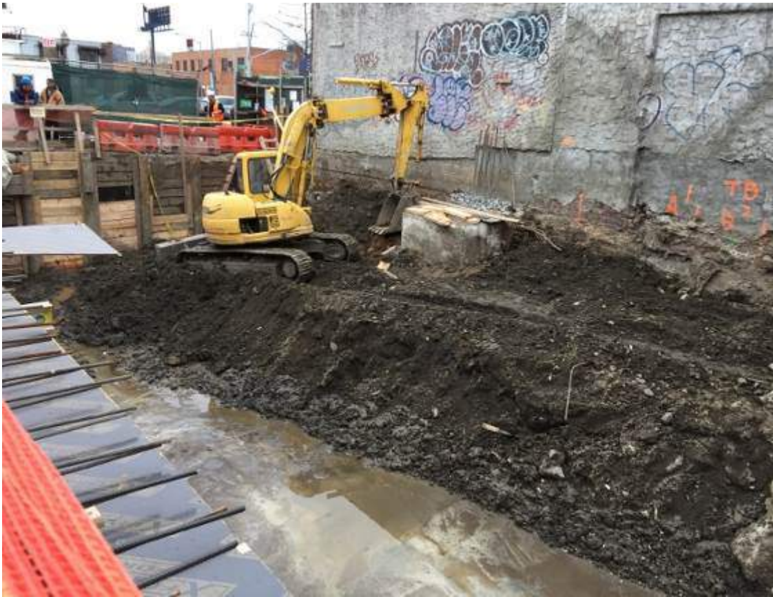
Photograph 113: View of the excavated area along the western portion of the site, facing west.
