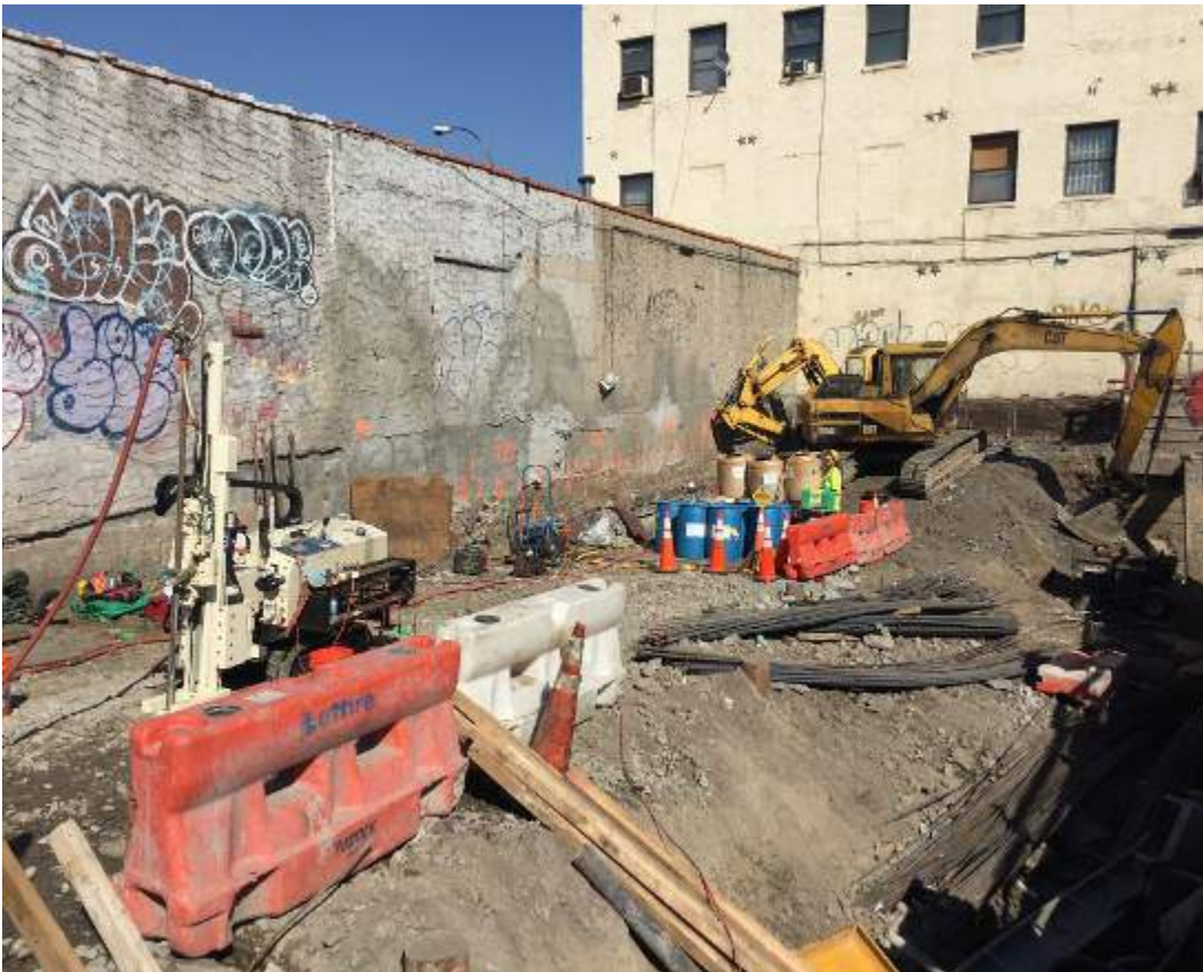
Photograph 94: View of the contained chemical storage and mixing area, facing north.
