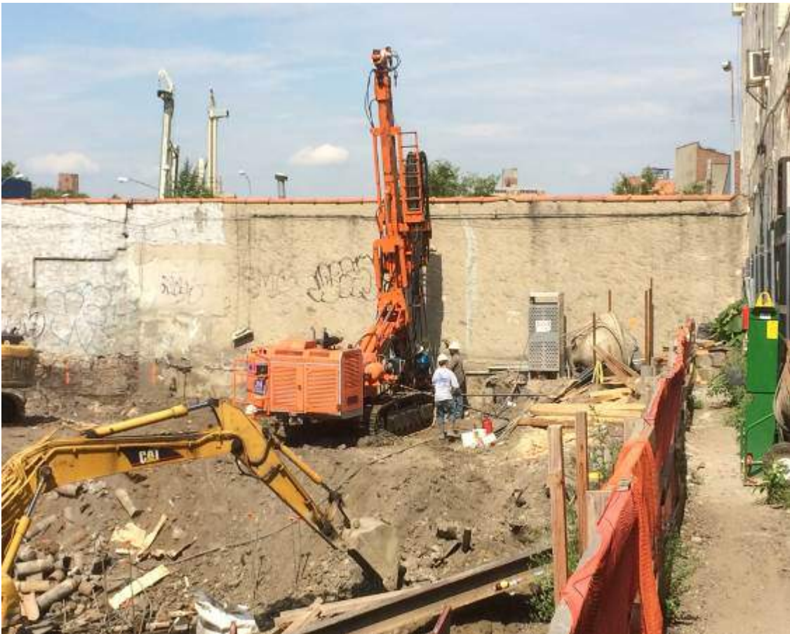
Photograph 84: View of the contractor drilling piles along the western boundary of the Site, facing west.
