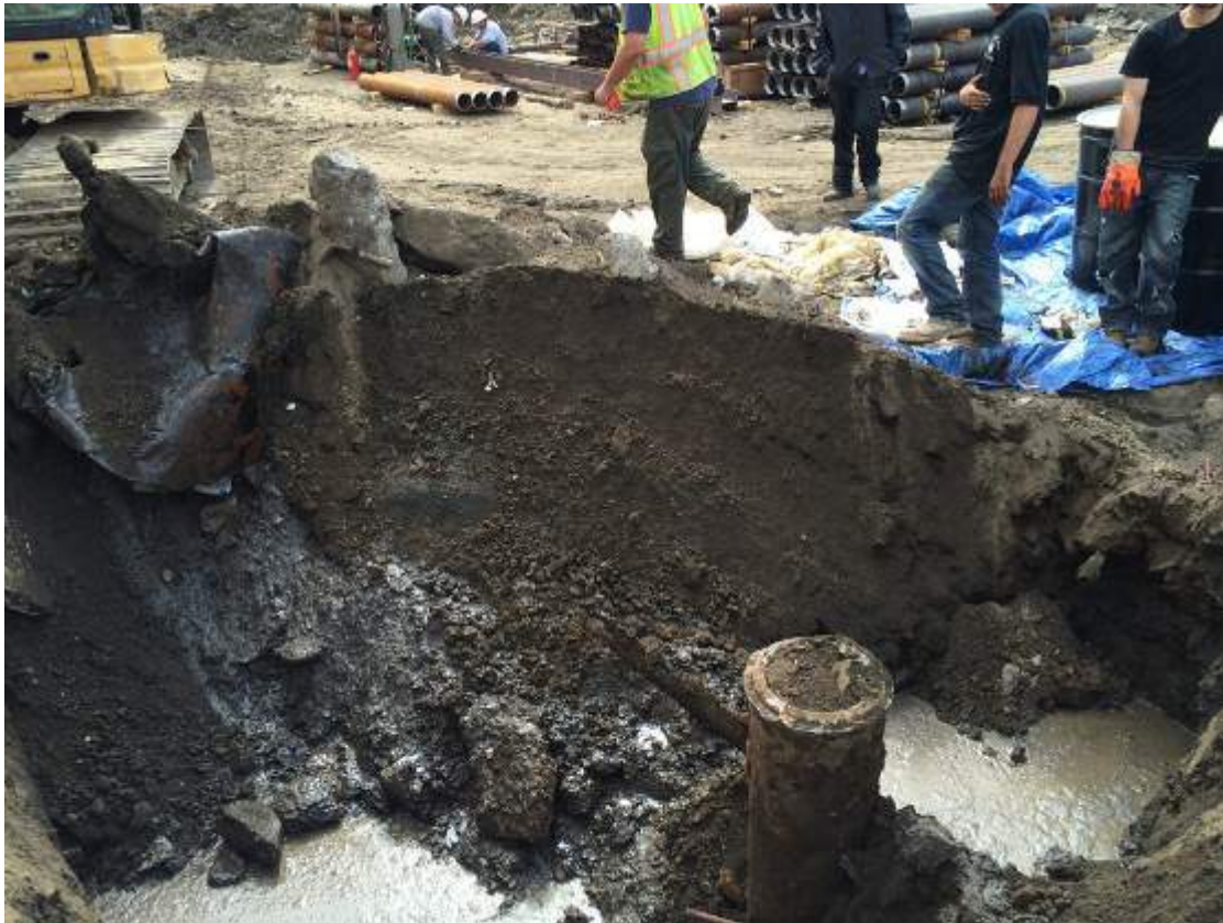
Photograph 29: View of the hydraulic Lift-2 discovered approximately five (5) feet east of Lift-1 and the location of where UST-18 and UST-19 were discovered.
