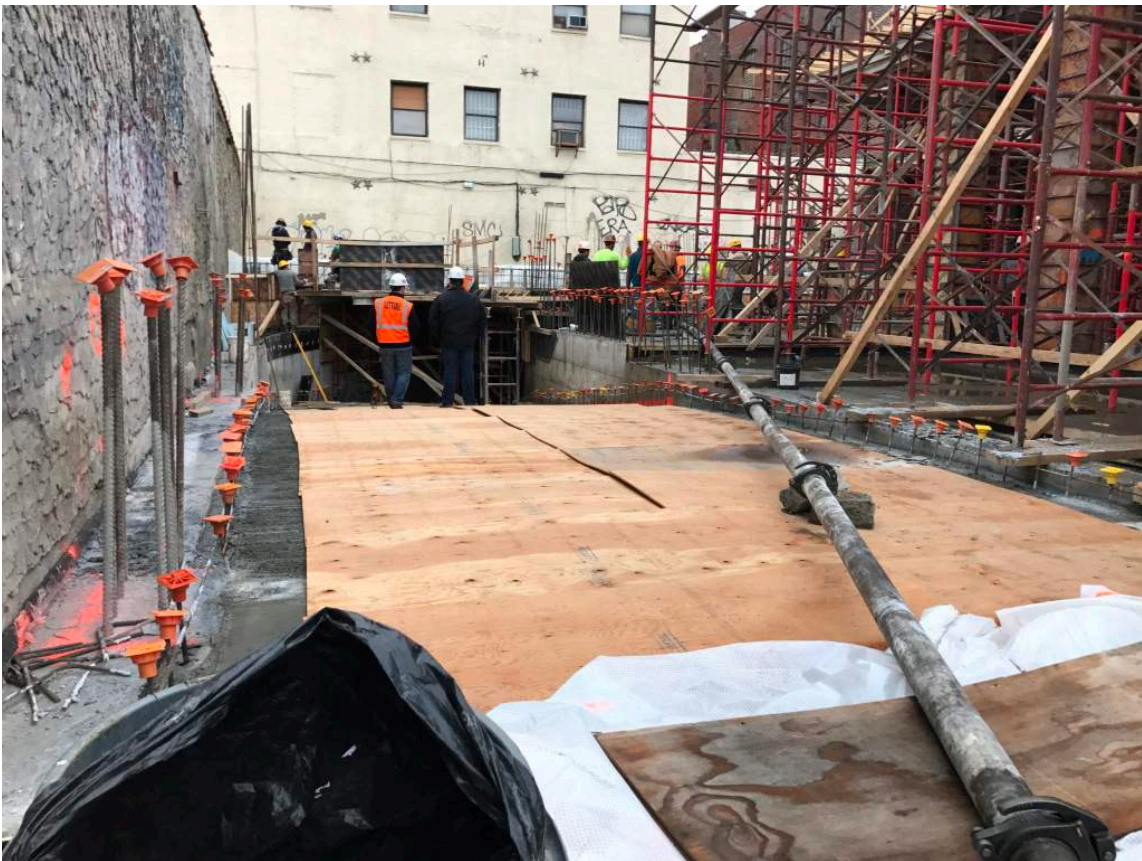
Photograph 132: View of the Site in preparation for the first floor concrete installation in the northern portion of the Site, facing northeast.
