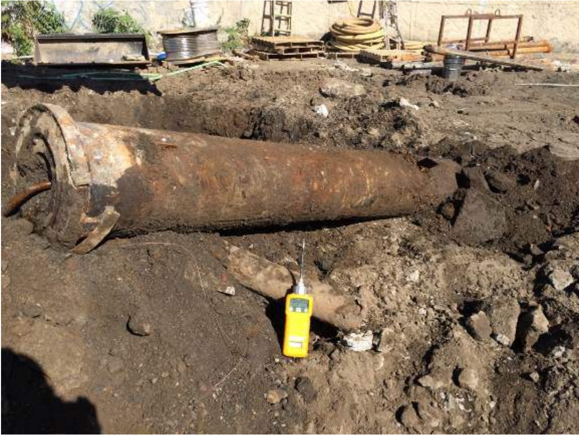
Photograph 25: View of the hydraulic Lift-1, discovered while excavating in the western portion of the Site.
