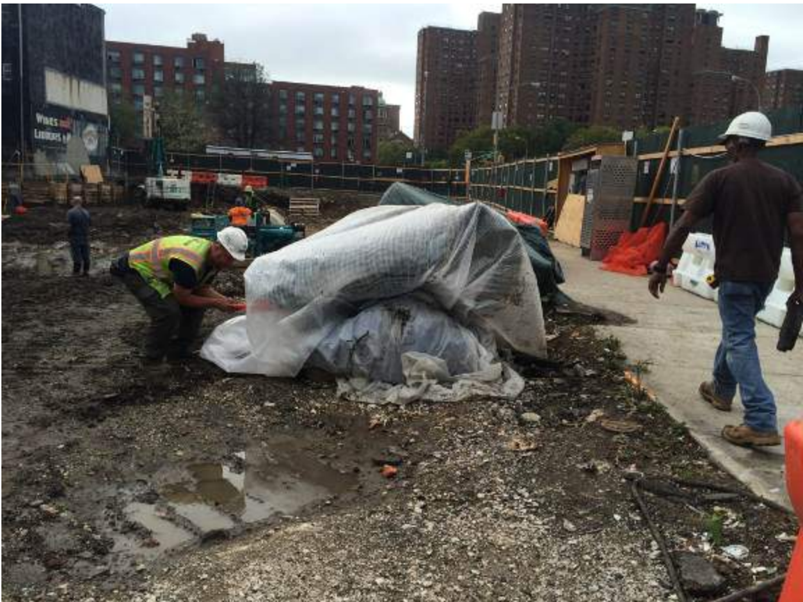
Photograph 22: View of the removed USTs (UST-16 and UST-17) covered in polyethylene sheeting.
