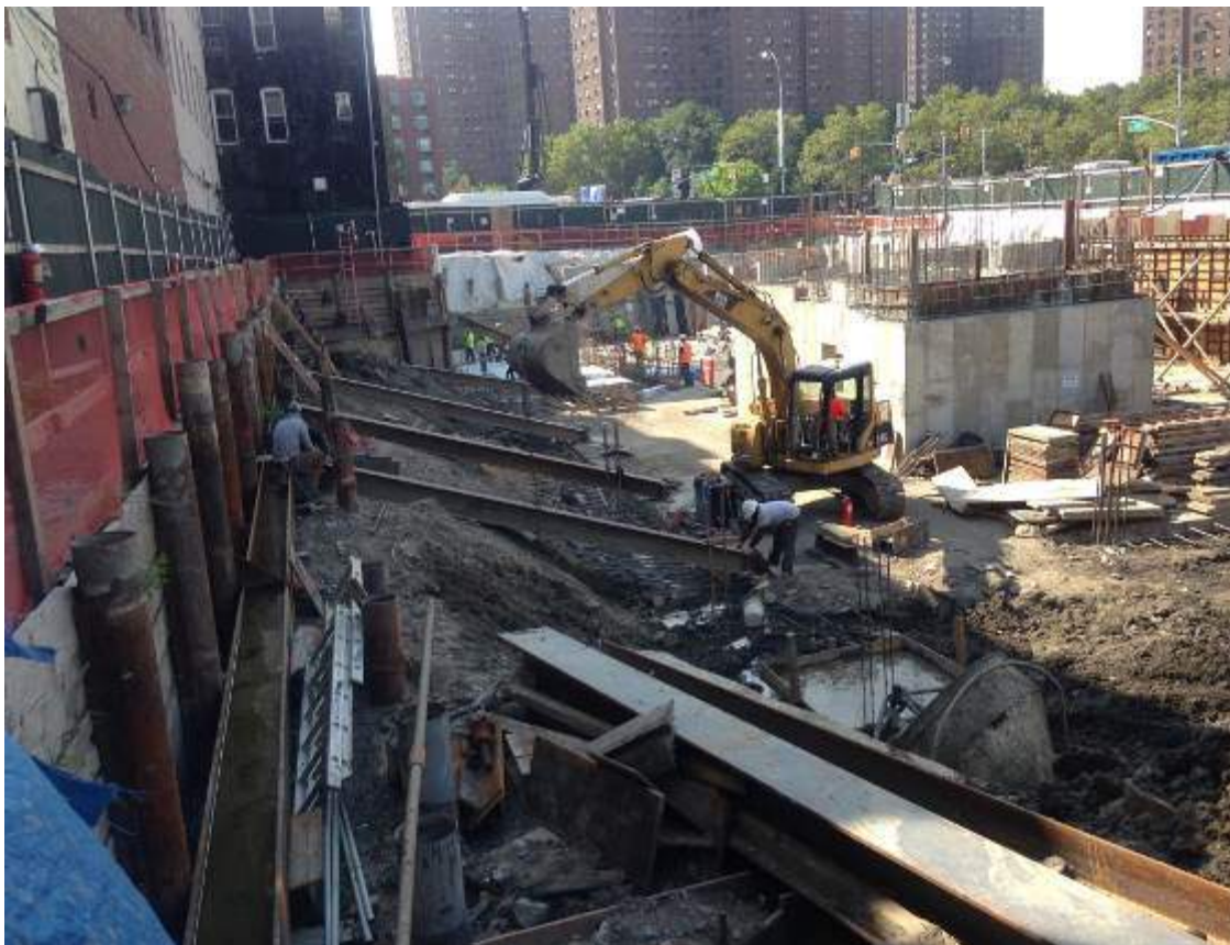
Photograph 68: View of the raker installation along the northern boundary of the site, facing southeast.
