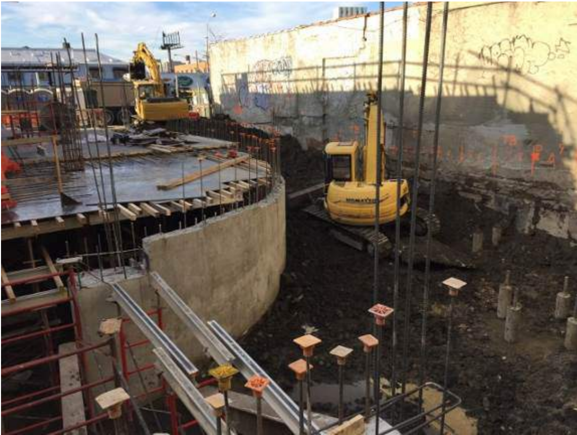
Photograph 119: View of the contractor directly loading soil for off-site disposal, facing west.
