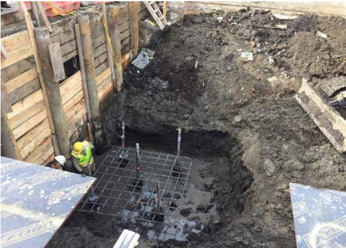
Photograph 118: View of the contractor installing rebar for the pile cap, facing southwest.
