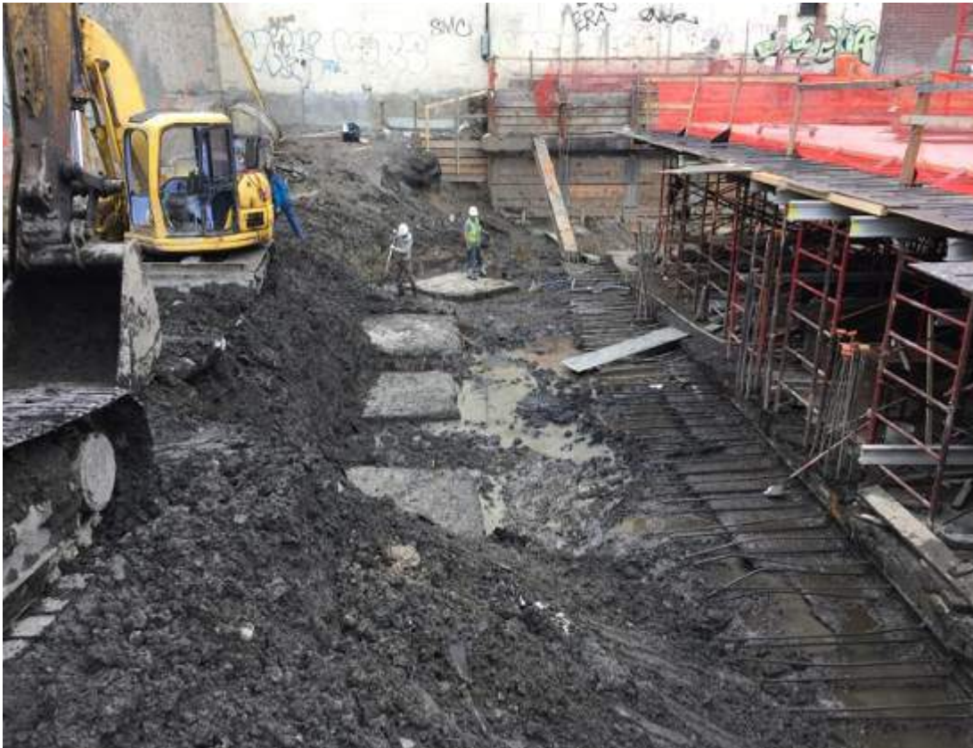
Photograph 109: View of the installed pile caps along the western portion of the site, facing northeast.
