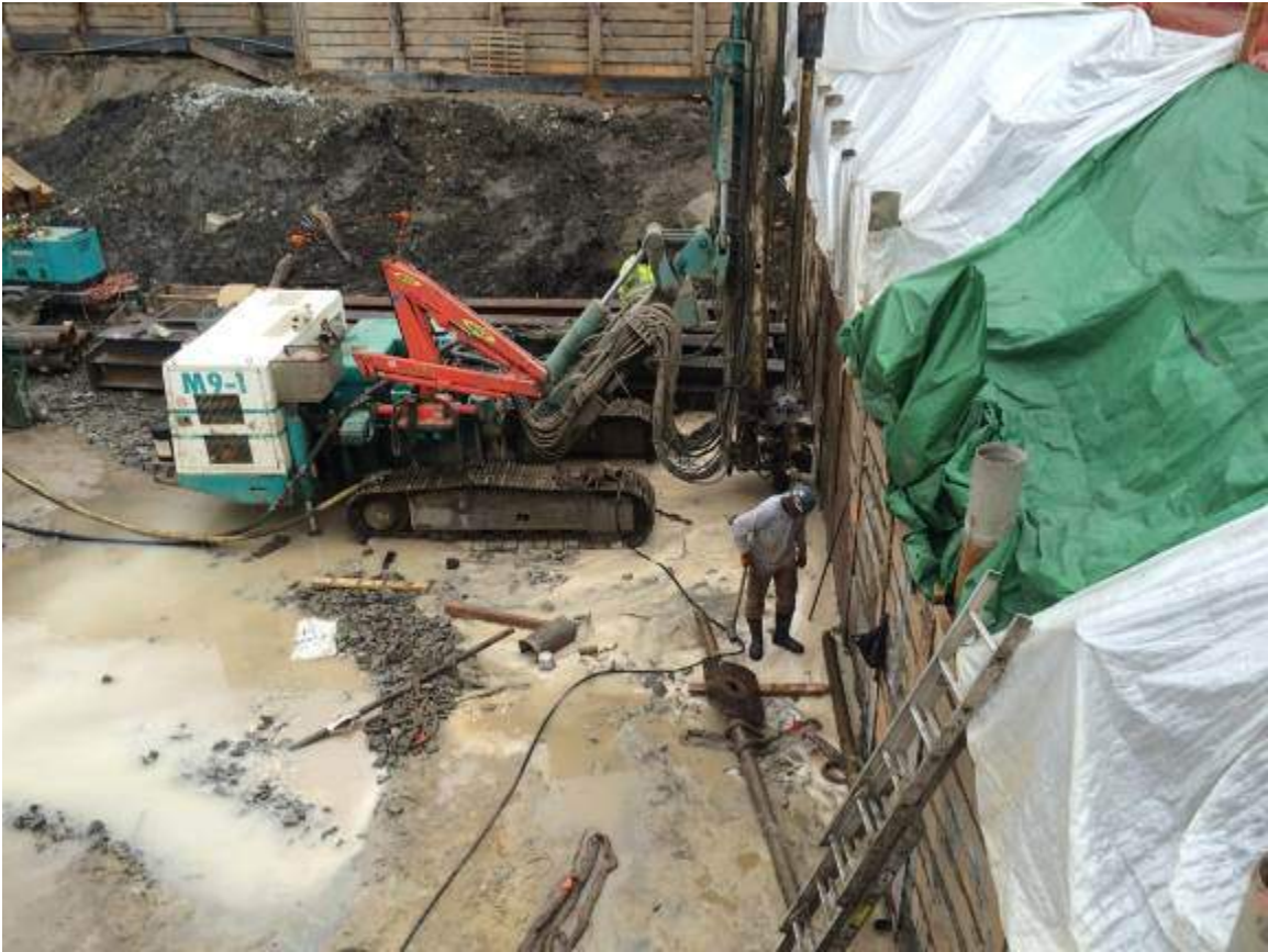
Photograph 43: View of the subcontractor installing piles along the eastern boundary of the Site.
