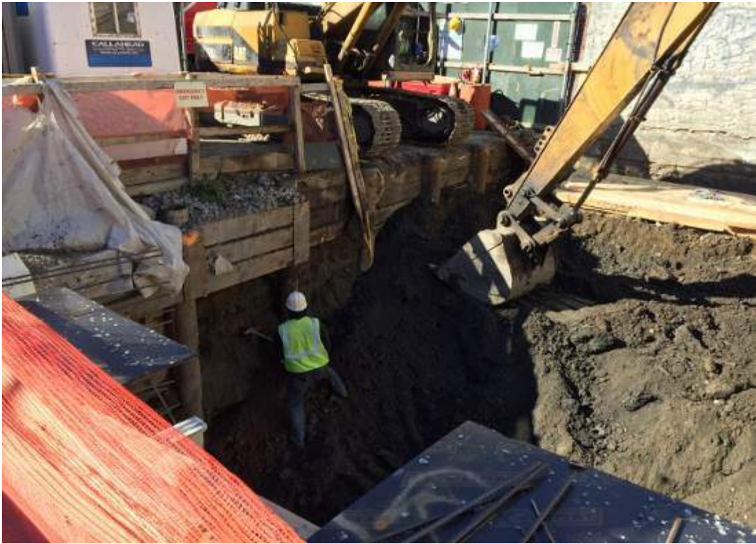
Photograph 111: View of the contractor preparing the south wall for lagging installation, facing west.
