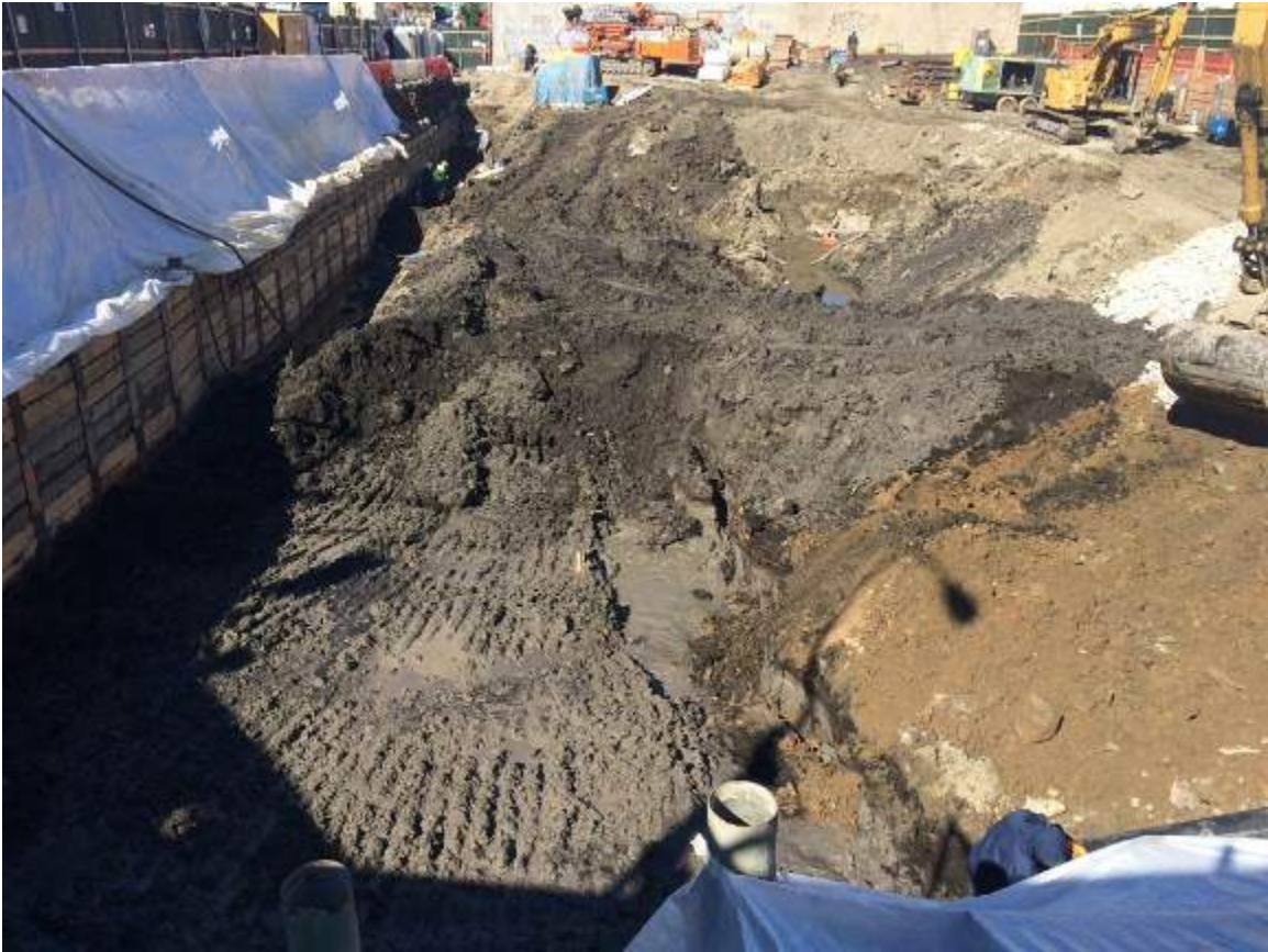
Photograph 33: View of the excavation area in the southern portion of the Site.
