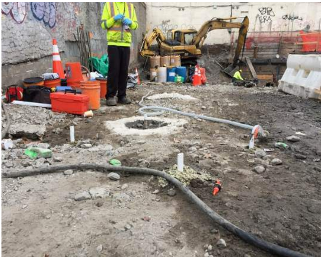
Photograph 100: View of the temporary injection well infrastructure, facing northeast.
