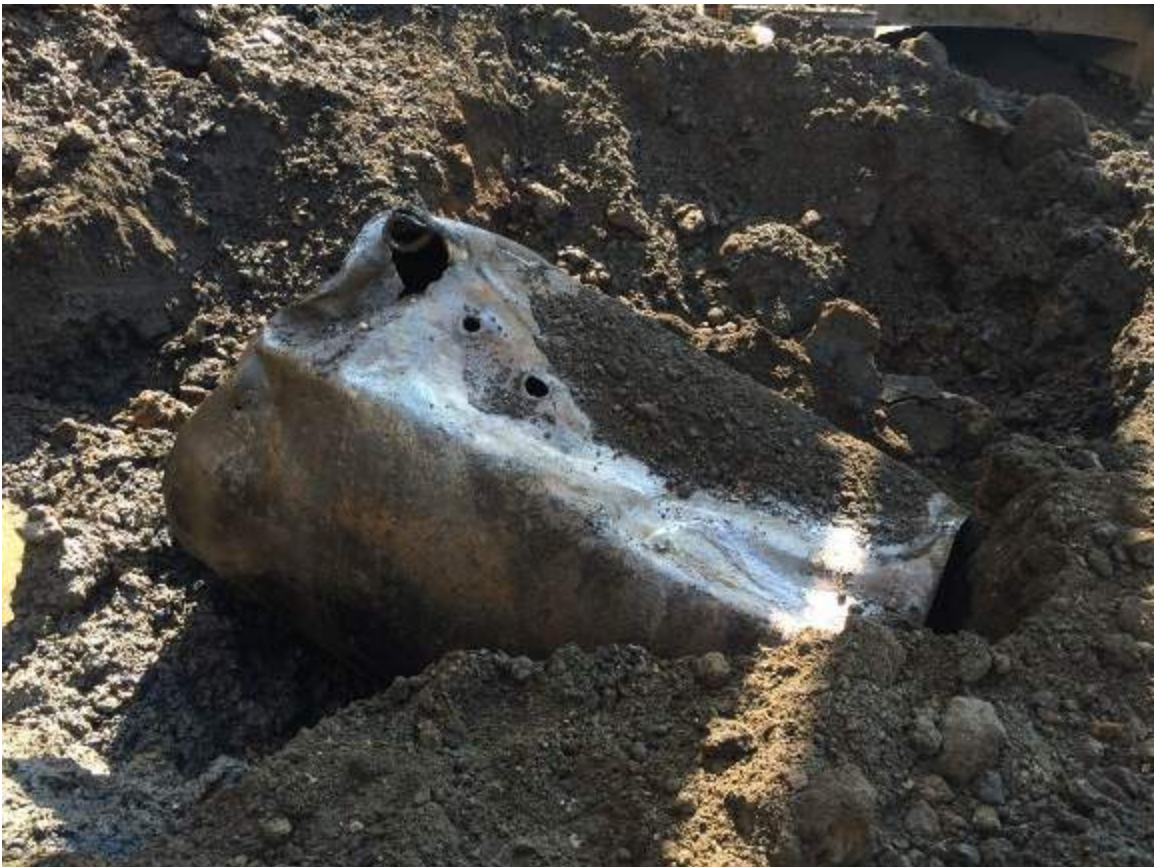
Photograph 18: View of UST-16 discovered along the northern boundary of the Site.
