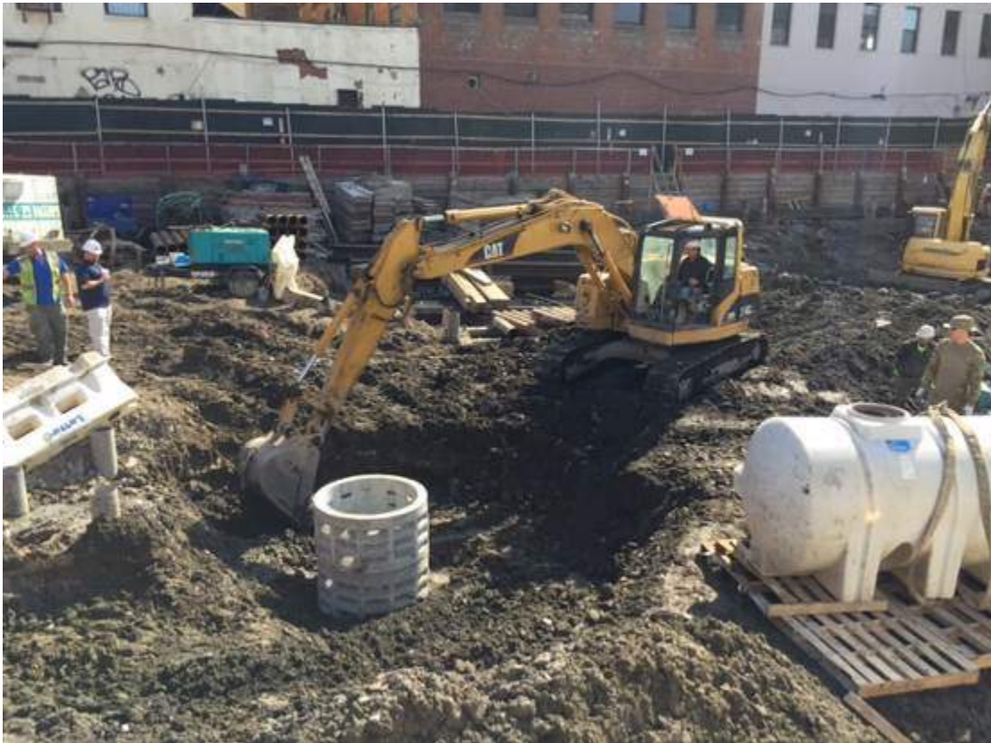
Photograph 53: View of the contractor excavating soil for the installation of a dewatering sump pit, facing northeast.
