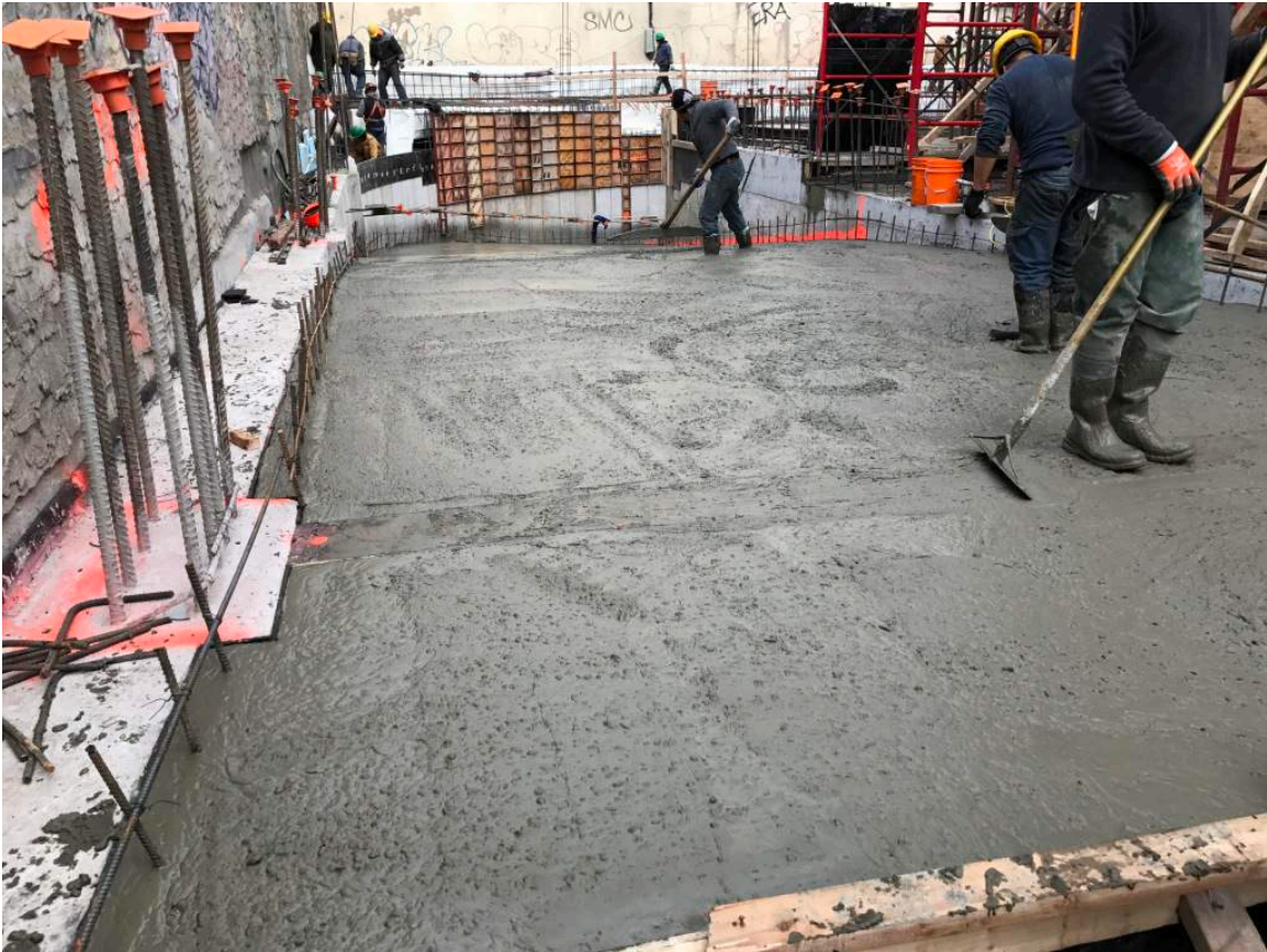
Photograph 131: View of the installed concrete in the southern portion of the ramp, facing north.
