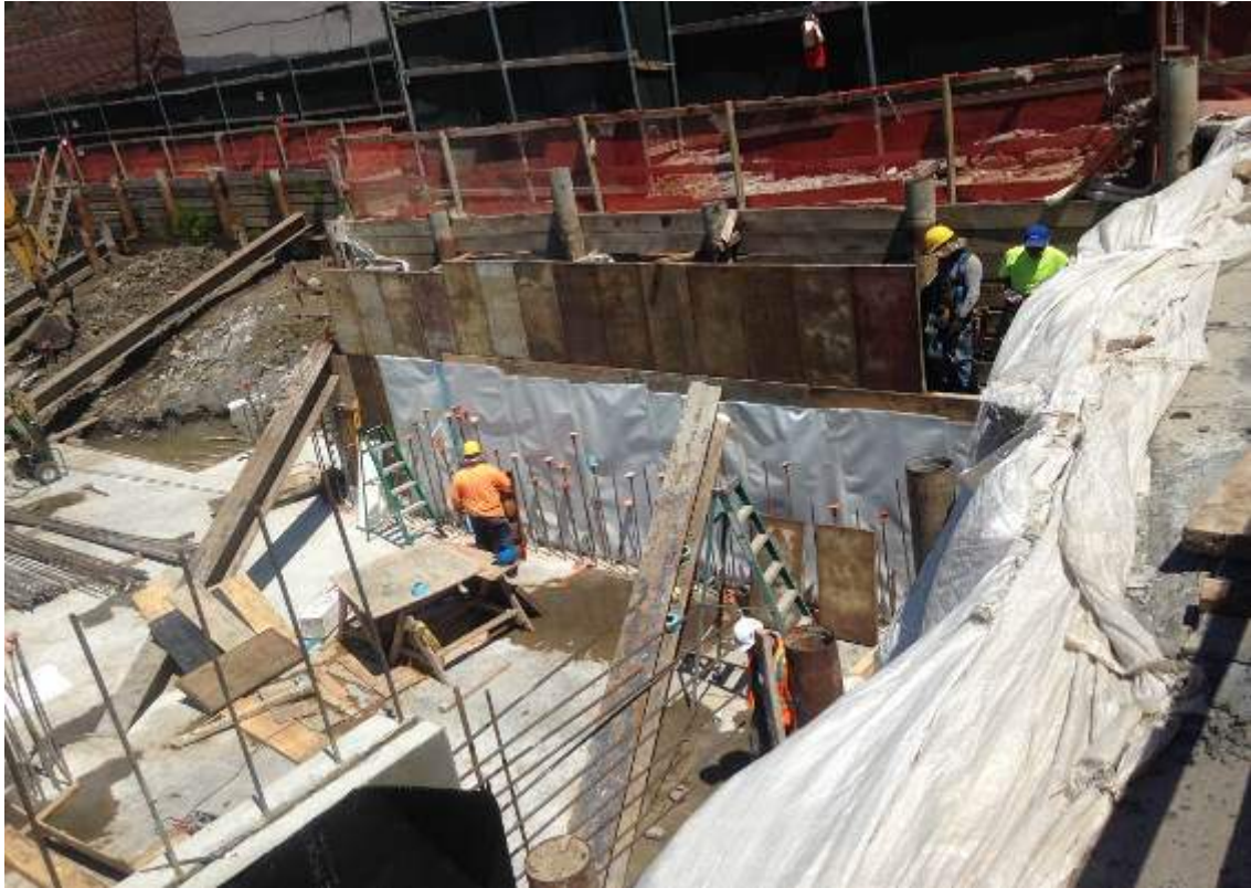
Photograph 71: View of the Preprufe 300R waterproofing membrane installation along the northeast boundary the site, facing north.
