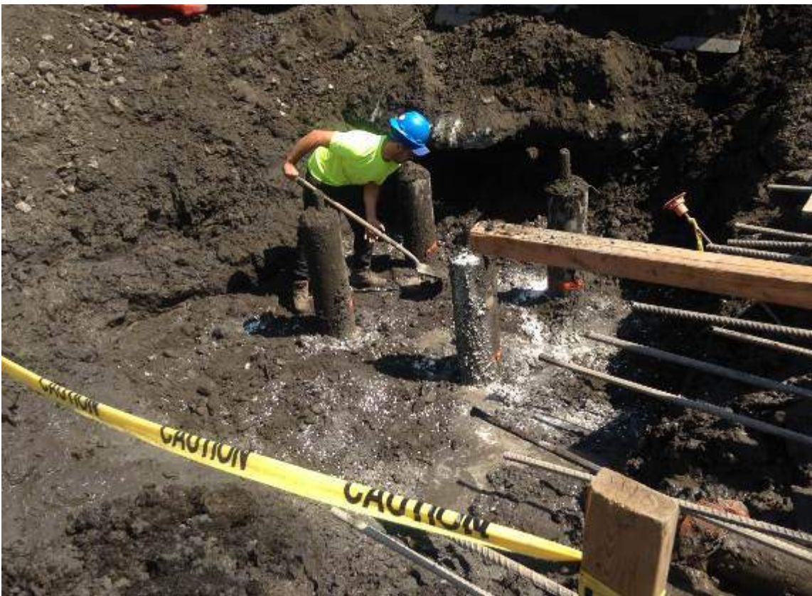
Photograph 66: View of the contractor hand-mixing ORC into the soil at the base of the pile cap excavation.
