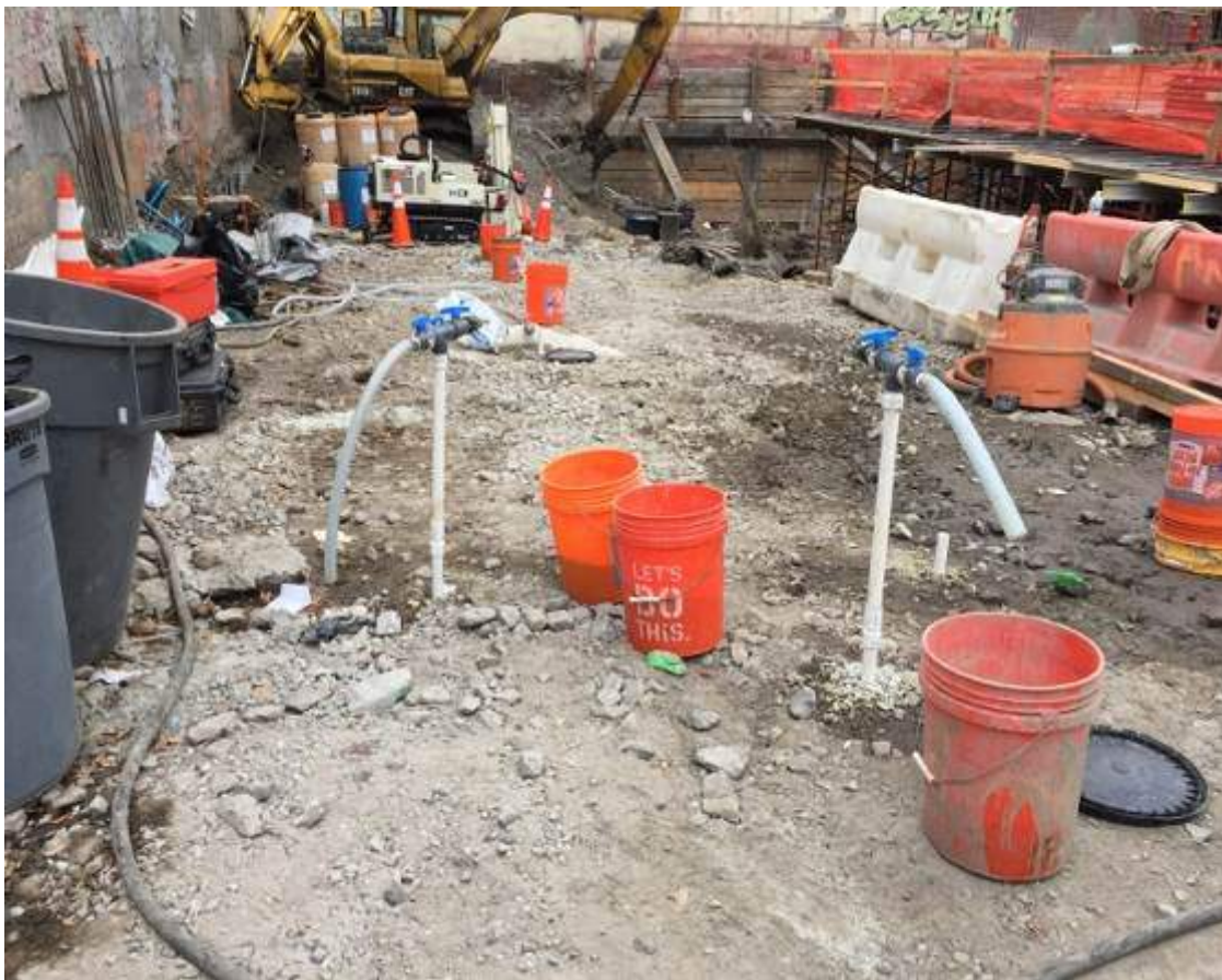
Photograph 99: View of the temporary gravity-feed injection well points TP-7 and TP-8, facing northeast.
