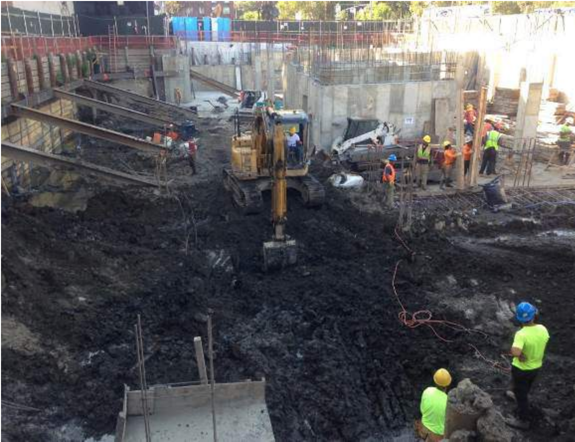
Photograph 75: View of the contractor excavating material in the western portion of the Site for the installation of a grade beam, facing east.
