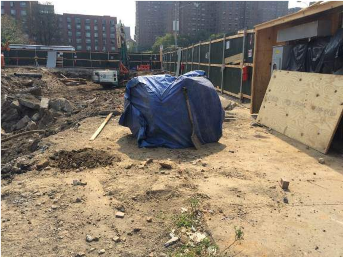
Photograph 14: View of UST-14 removed and covered in plastic along the E. 138 th Street boundary.
