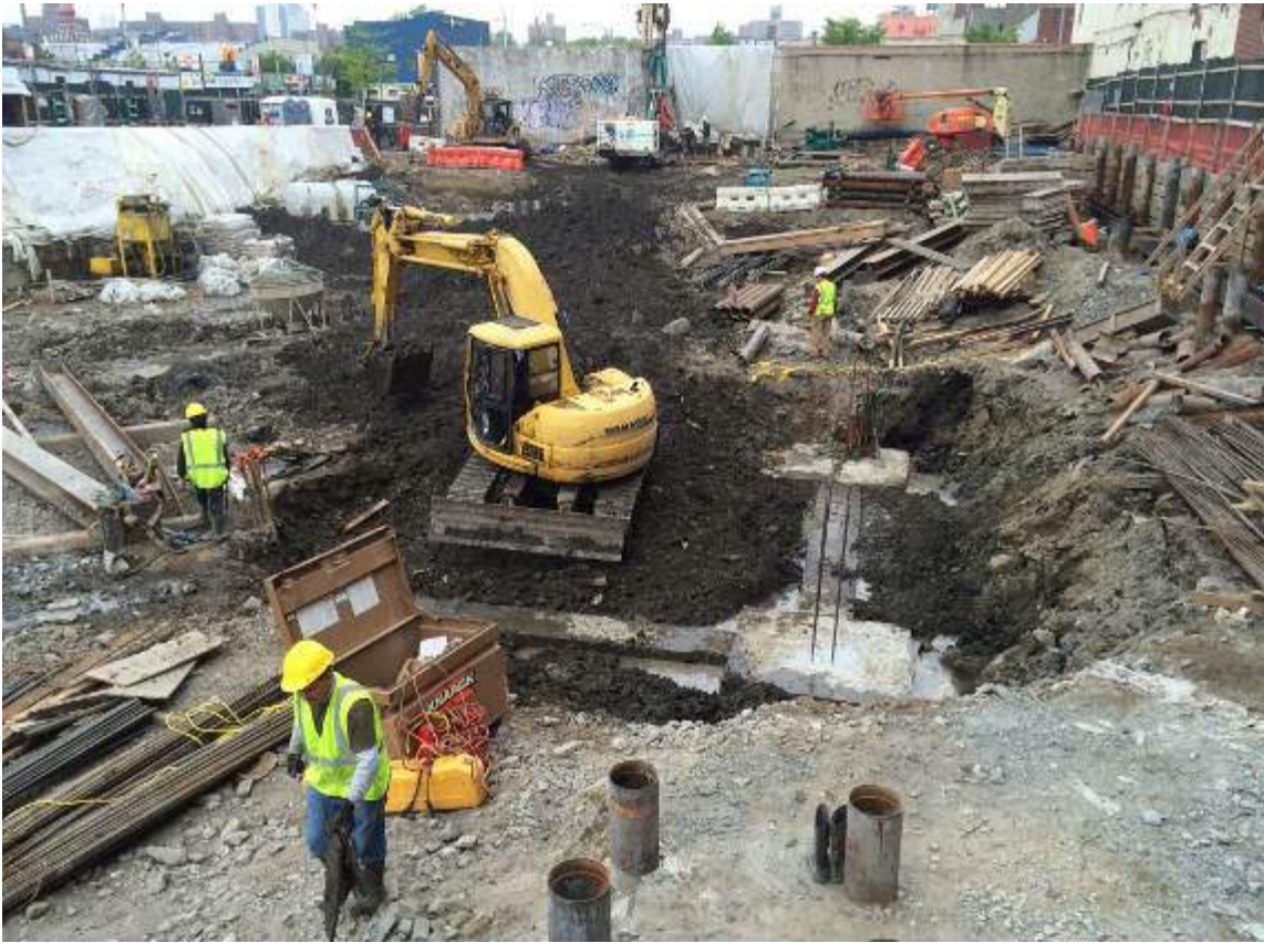
Photograph 55: View of the installed grade beams and pile caps along the northern boundary of the Site, facing northwest.
