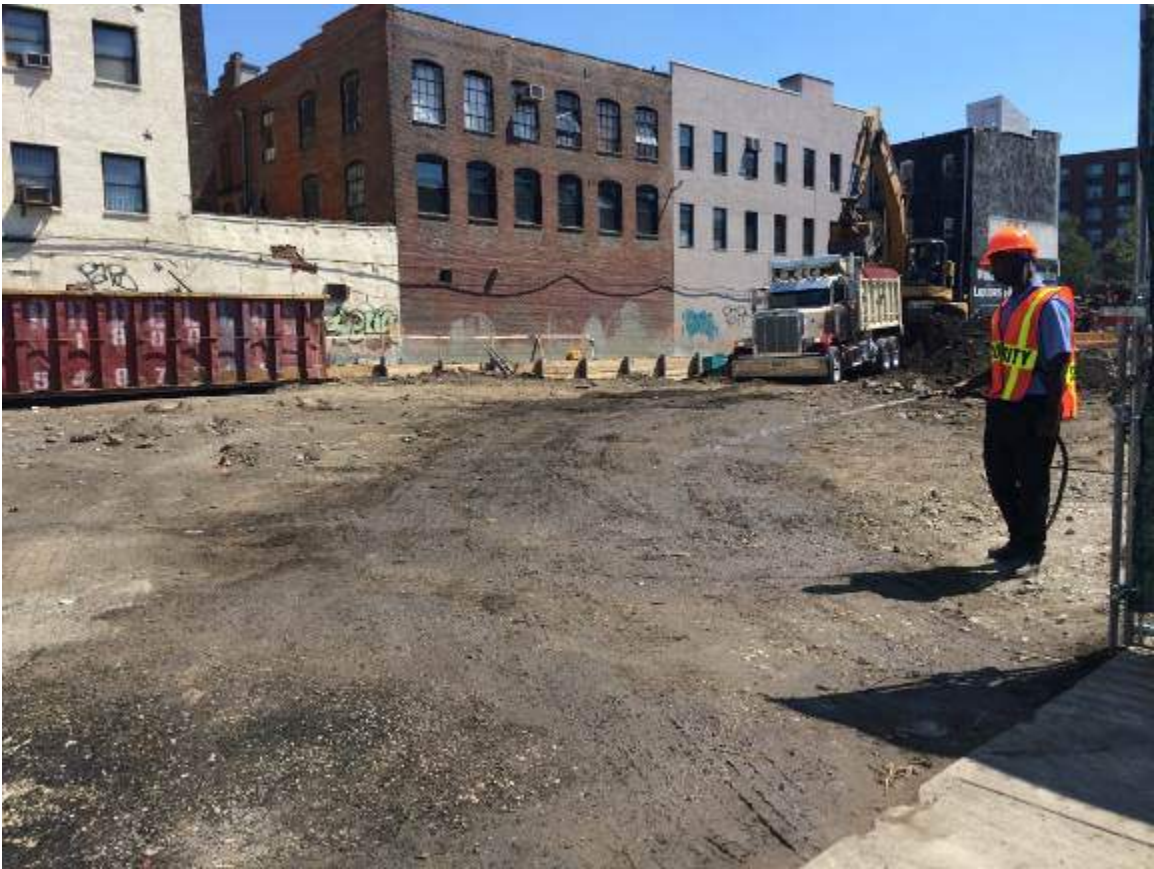
Photograph 5: View of the contractor applying water to the Site entrance area, facing east.
