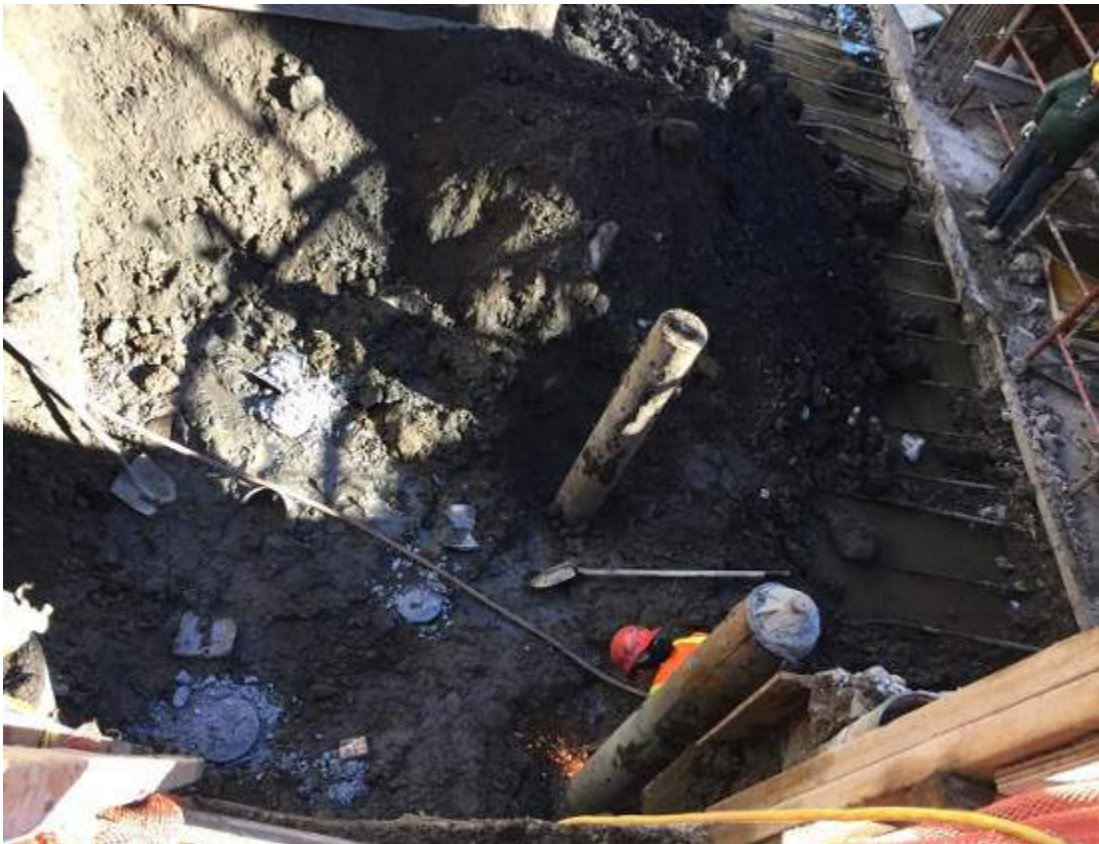
Photograph 112: View of the contractor welding piles along the southern boundary of the site.
