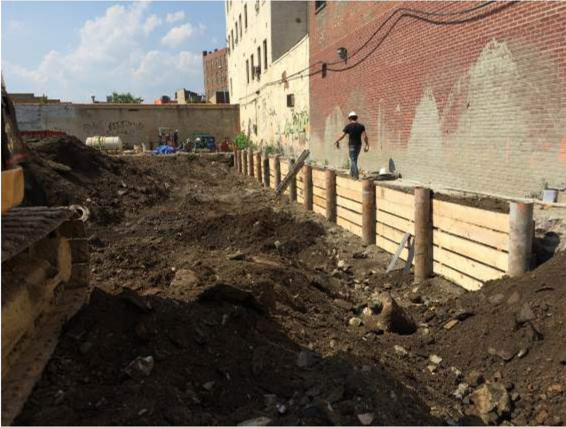
Photograph 7: View of the lagging installation along the northern boundary of the Site, facing north.
