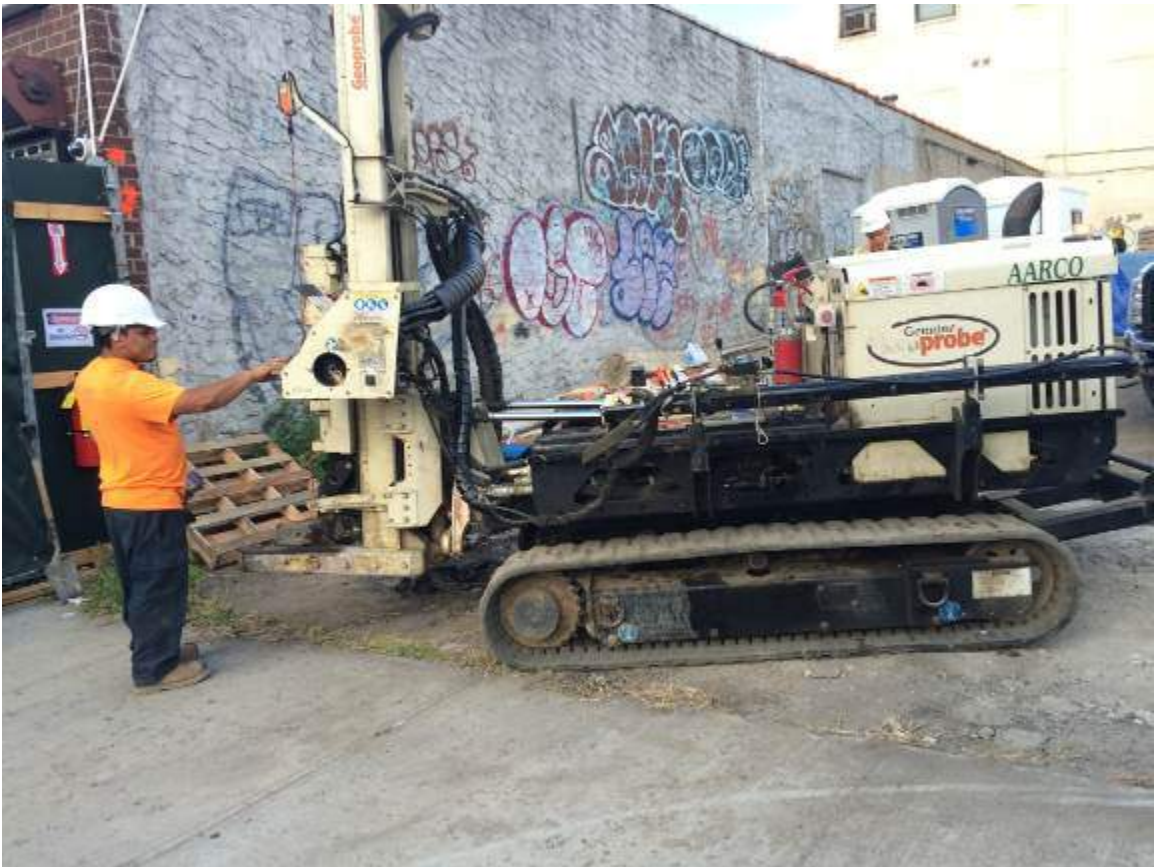
Photograph 1: View of AARCO Environmental Services Corp. installing a temporary monitoring well in the sidewalk along E. 138 th Street prior to the start of remediation, facing north.
