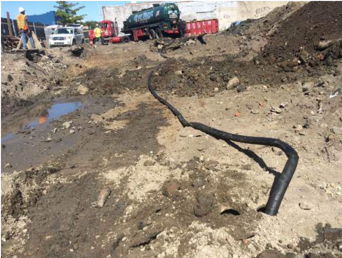
Photograph 8: View of Mercury Tank Cleaners removing the liquid contents from the USTs.
