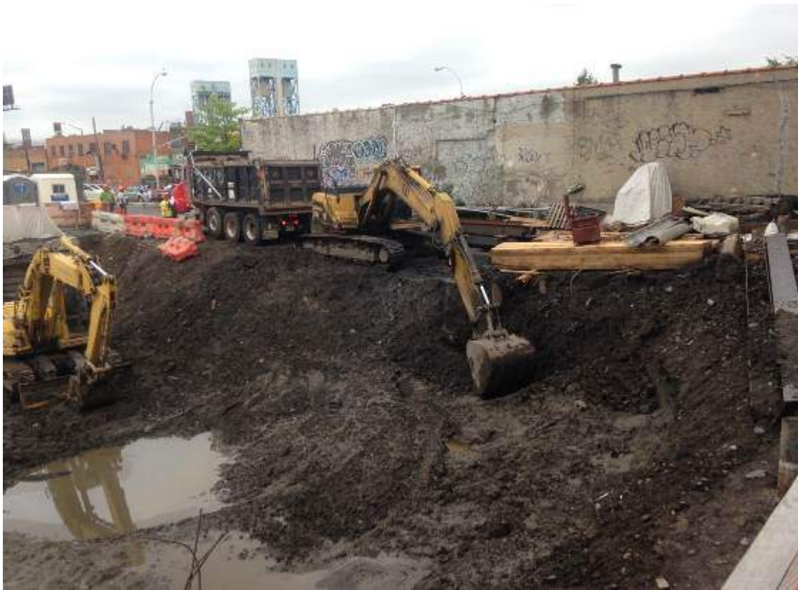
Photograph 73: View of the contractor excavating material for off-site disposal in the northwestern portion of the Site, facing northwest.
