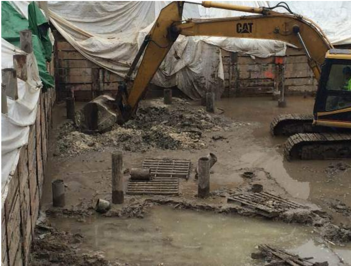
Photograph 47: View of the contractor excavating in the southern portion of the site in preparation for installing a pile cap, facing southwest.
