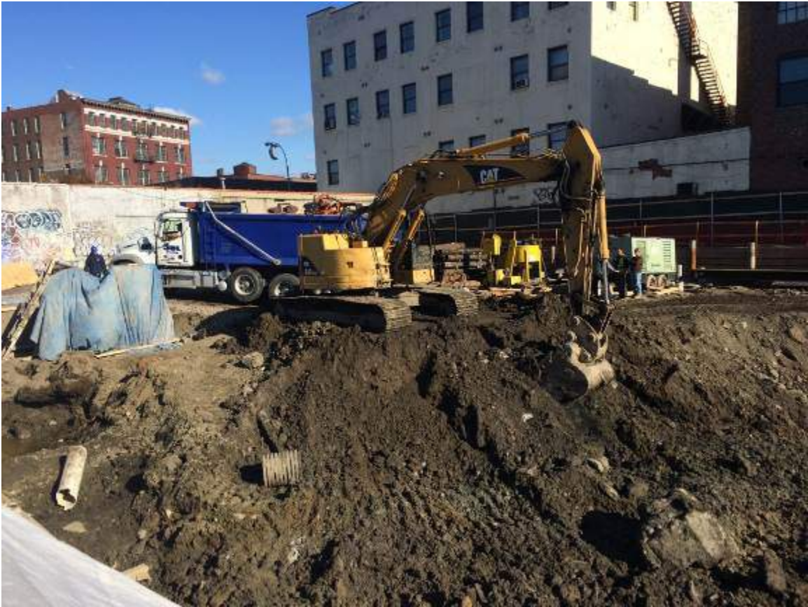
Photograph 31: View of the excavation area in the western portion of the Site.
