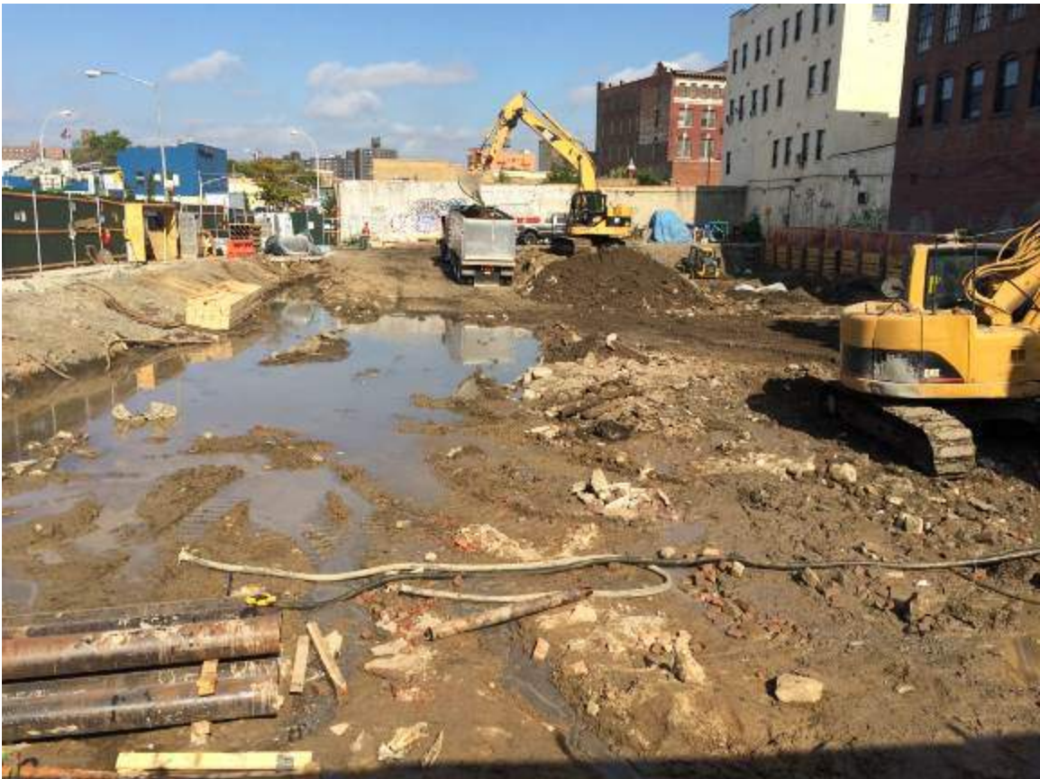
Photograph 20: View of the Site and the contractor directly loading material for off-site disposal, facing west.
