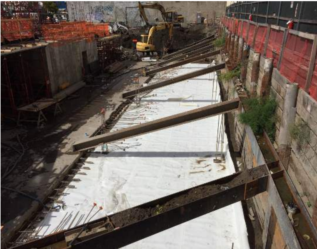
Photograph 88: View of the installed waterproofing membrane along the northern boundary of the site, facing northwest.
