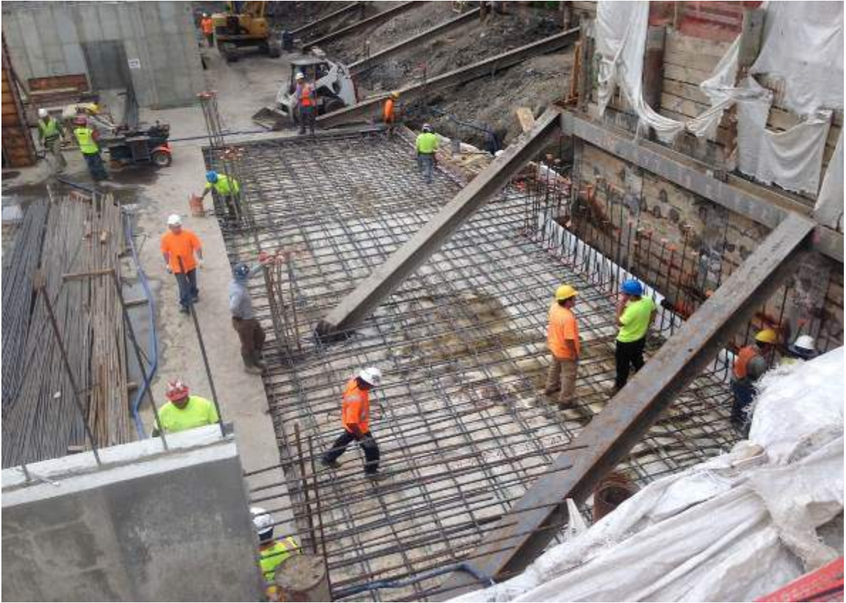
Photograph 69: View of the contractor installing rebar in the northeast corner of the site.
