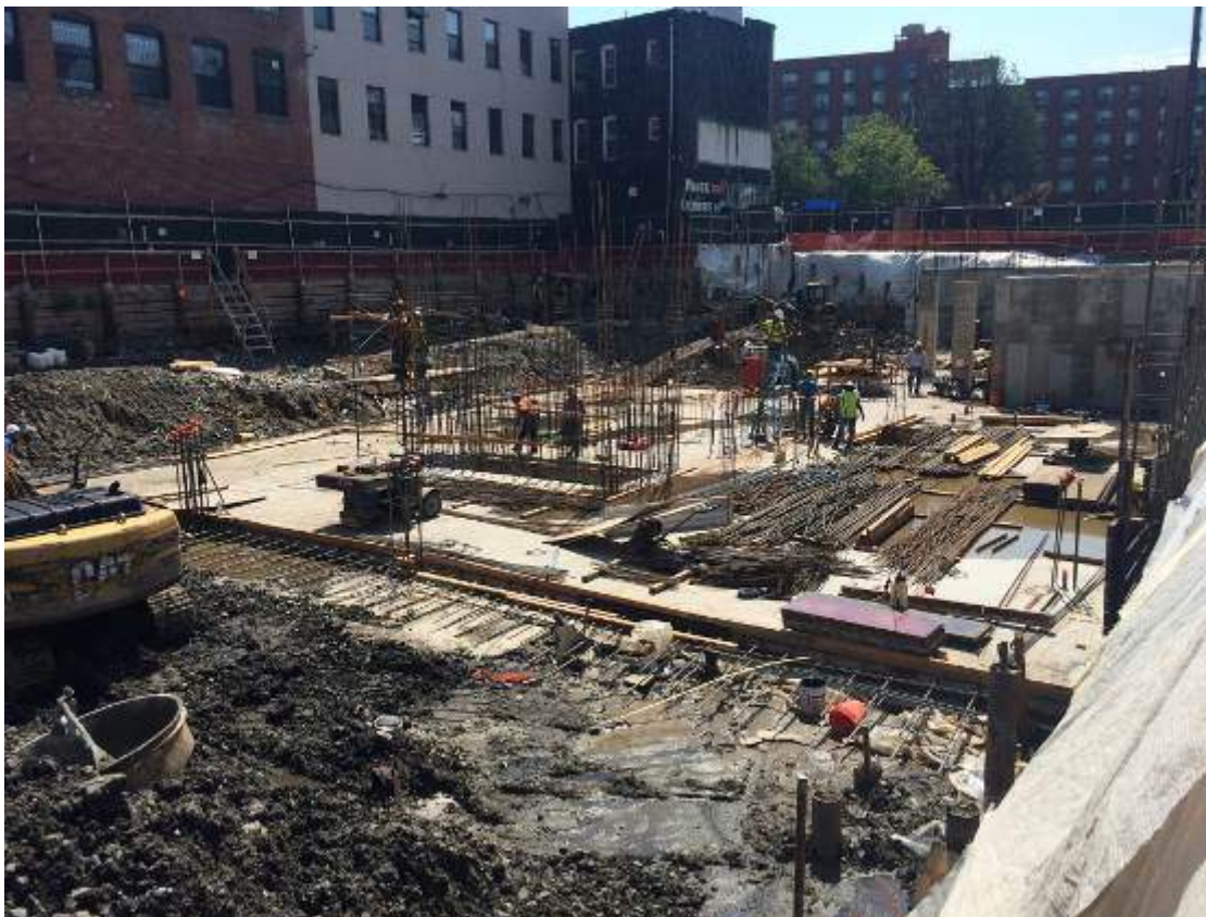
Photograph 63: View of the installed foundation slab in the central portion of the Site, facing east.
