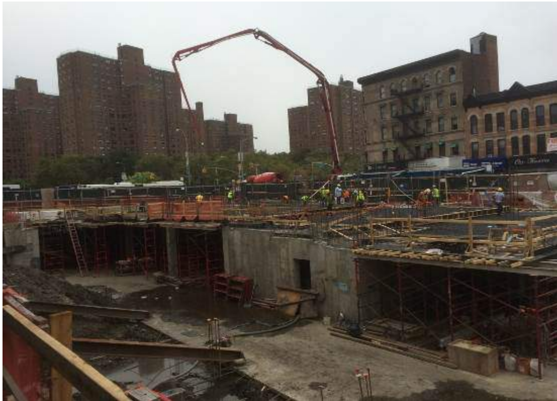
Photograph 86: View of the contractor installing the first floor in the southeastern and central portions of the Site, facing southeast.
