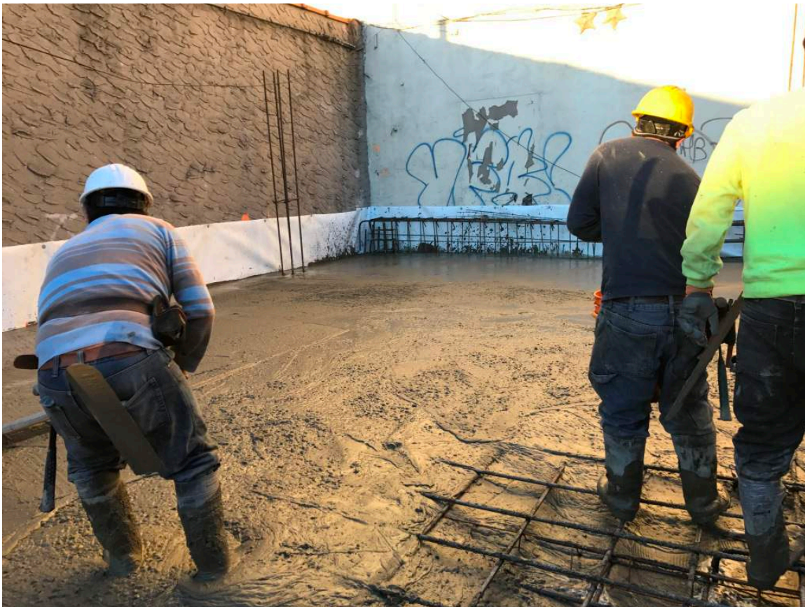
Photograph 138: Additional view of the concrete installation in the northern corner of the Site, facing north.
