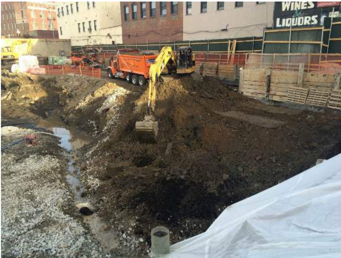
Photograph 37: View of the excavation area in the northern portion of the Site, facing north.
