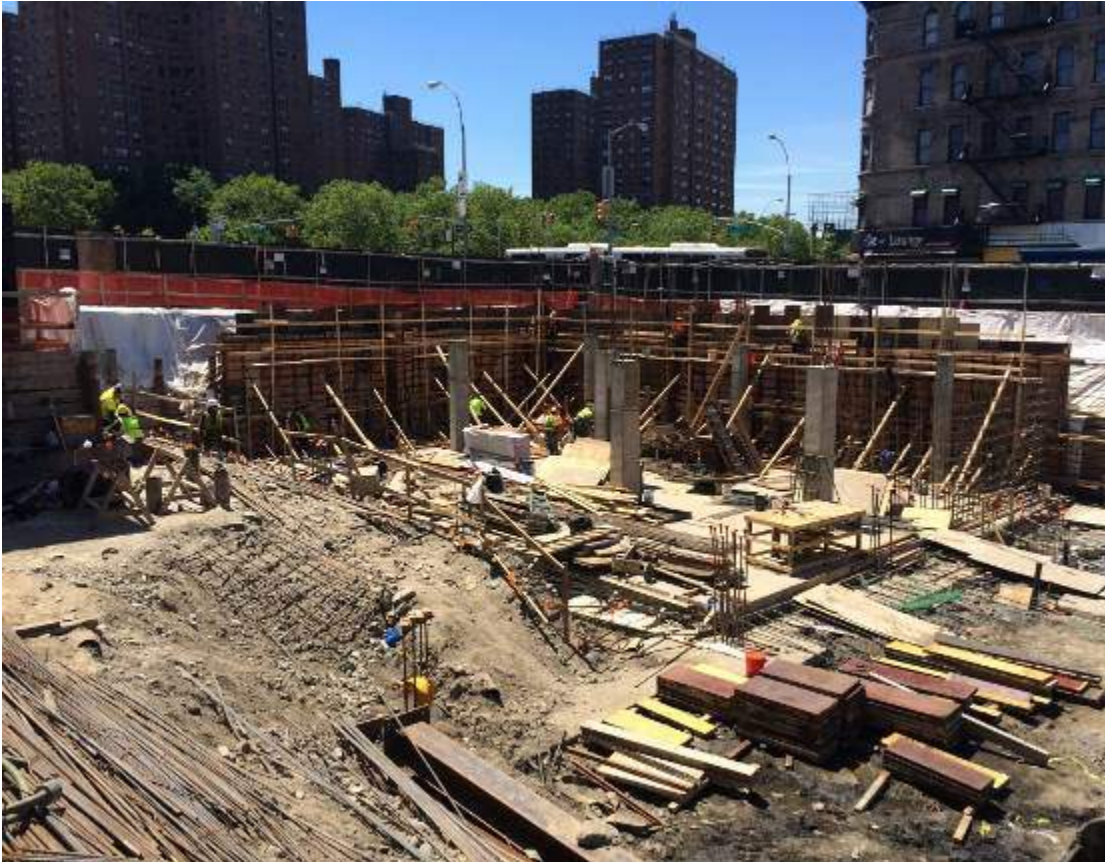
Photograph 59: View of the installed foundation slab and sidewall formwork in the southeastern corner of the Site, facing south.
