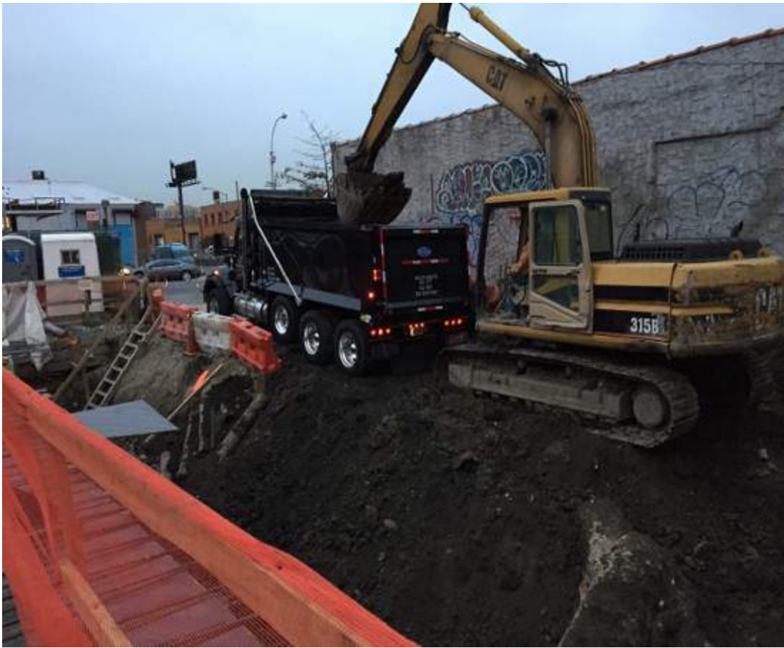
Photograph 103: View of the contractor directly loading soil for off-site disposal, facing west.
