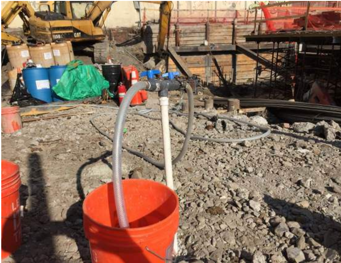
Photograph 98: View of one (1) of the one-inch gravity feed injection wells, facing east.
