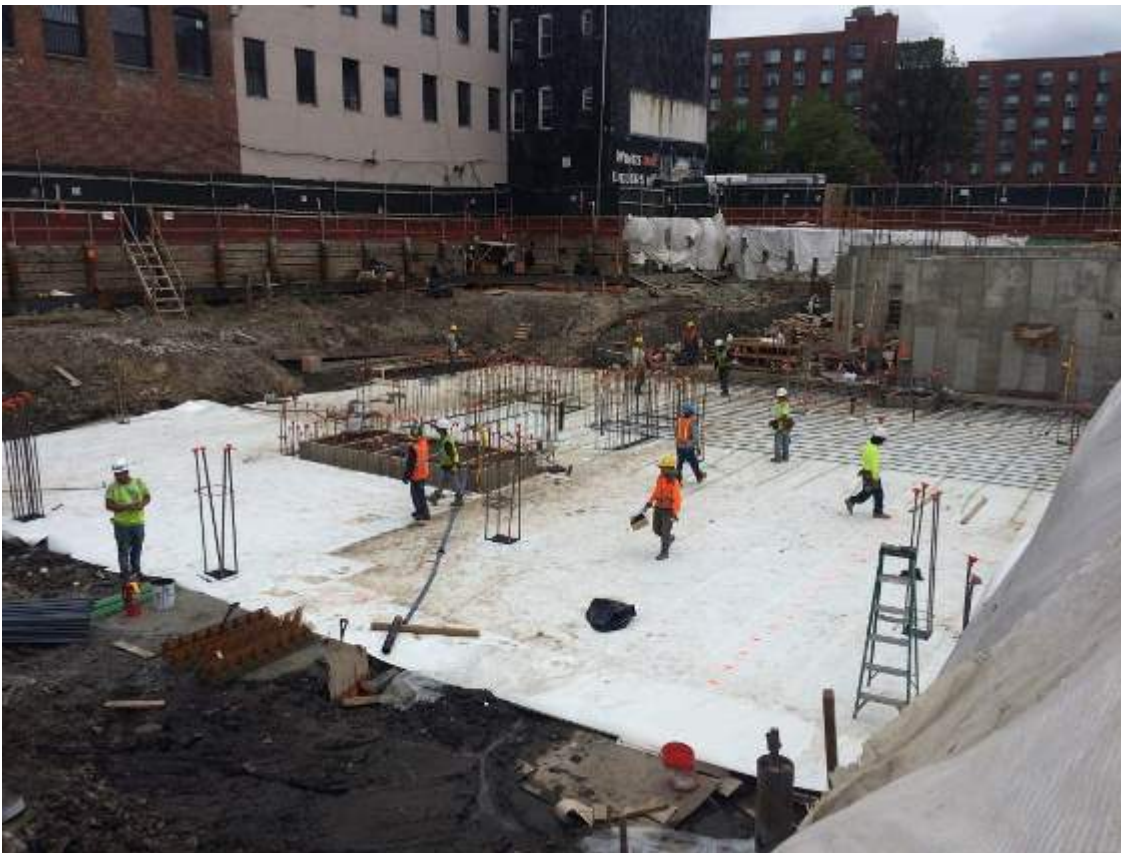
Photograph 62: View of the installed waterproofing membrane and rebar in the central portion of the Site, facing east.
