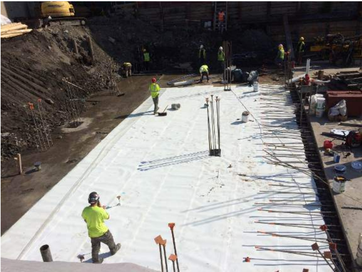
Photograph 79: View of the contractor installing the Preprufe 300R waterproofing membrane in the western portion of the Site, facing north.
