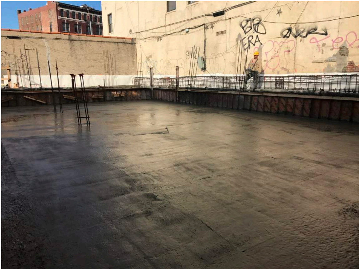
Photograph 134: View of the installed concrete in the northern portion of the Site for the first floor, facing north.
