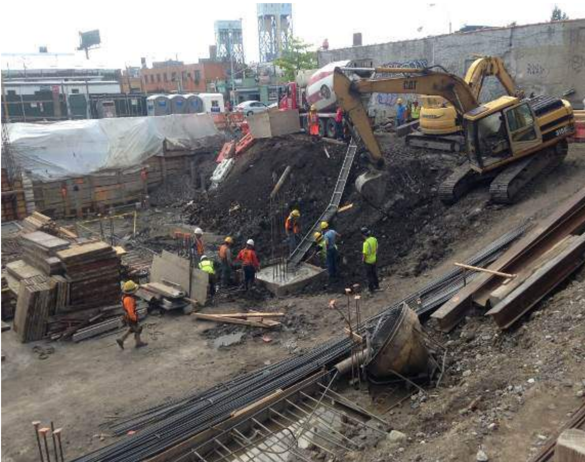
Photograph 65: View of the contractor pouring concrete into a pile cap, facing west.
