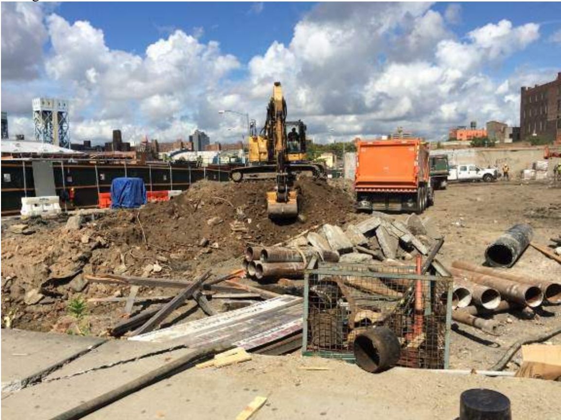
Photograph 2: View of the beginning of excavation in the southeast portion of the Site, facing northwest.
