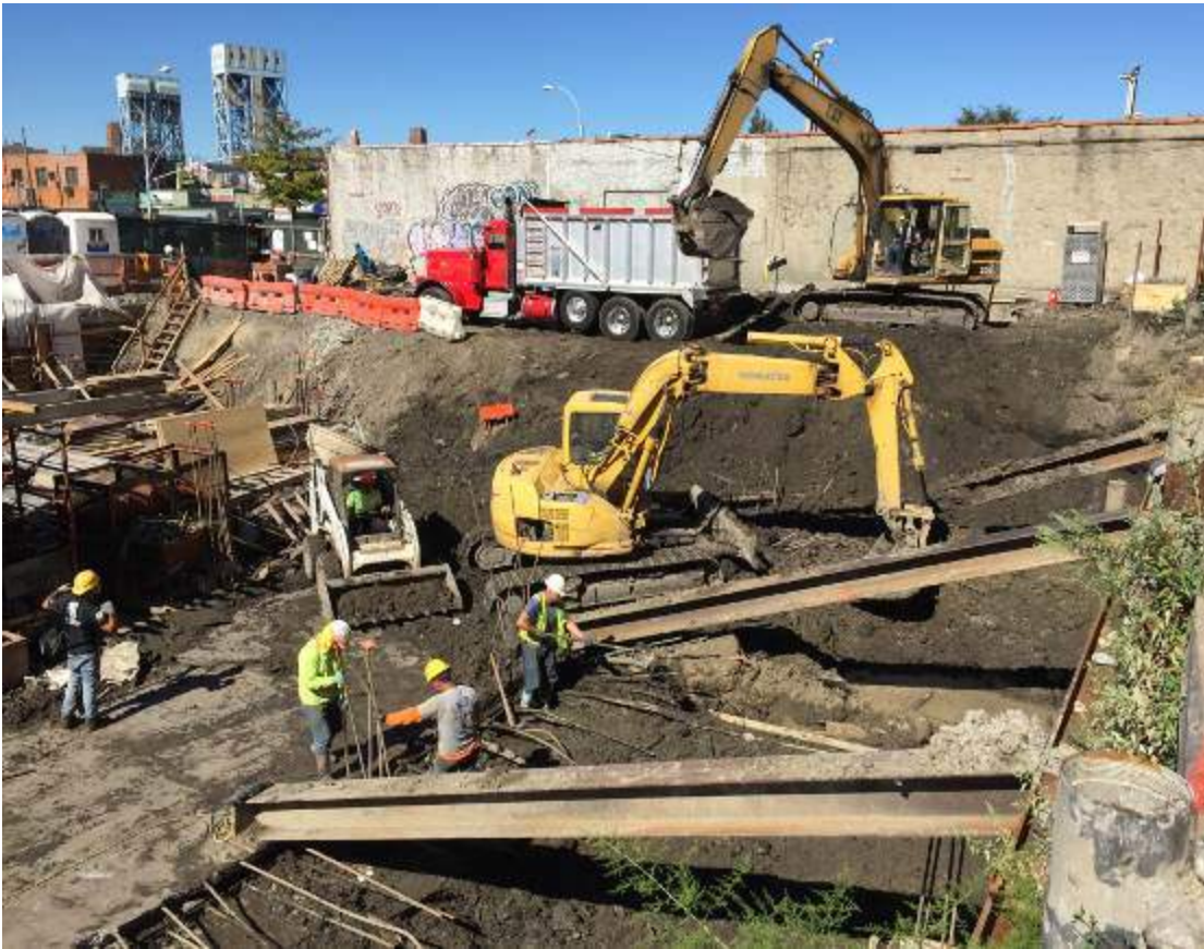
Photograph 87: View of the contractor excavating in the northwestern corner of the Site, facing northwest.
