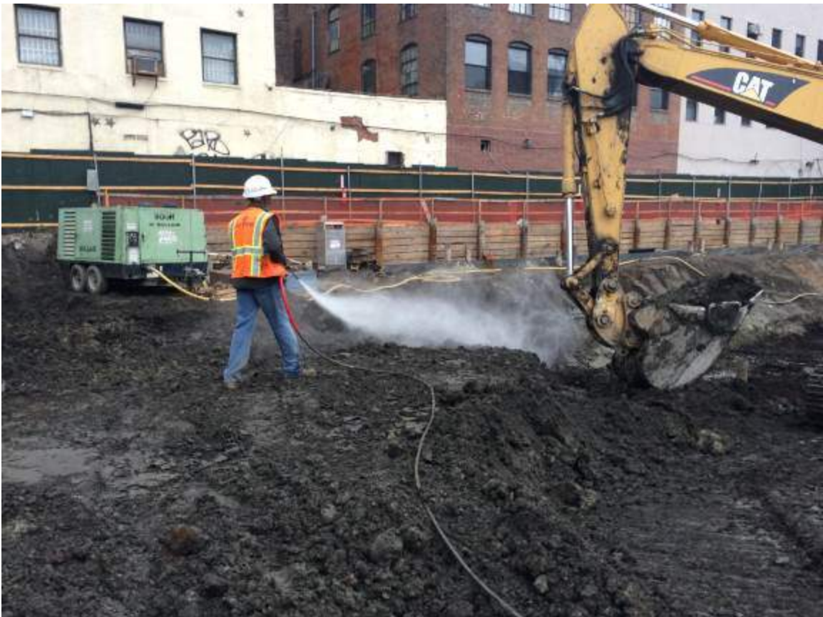
Photograph 44: View of the contractor using the Landa 3500 PSI Power Washer to apply the BioSolve ® Pinkwater vapor suppressant to the petroleum-impacted soil.
