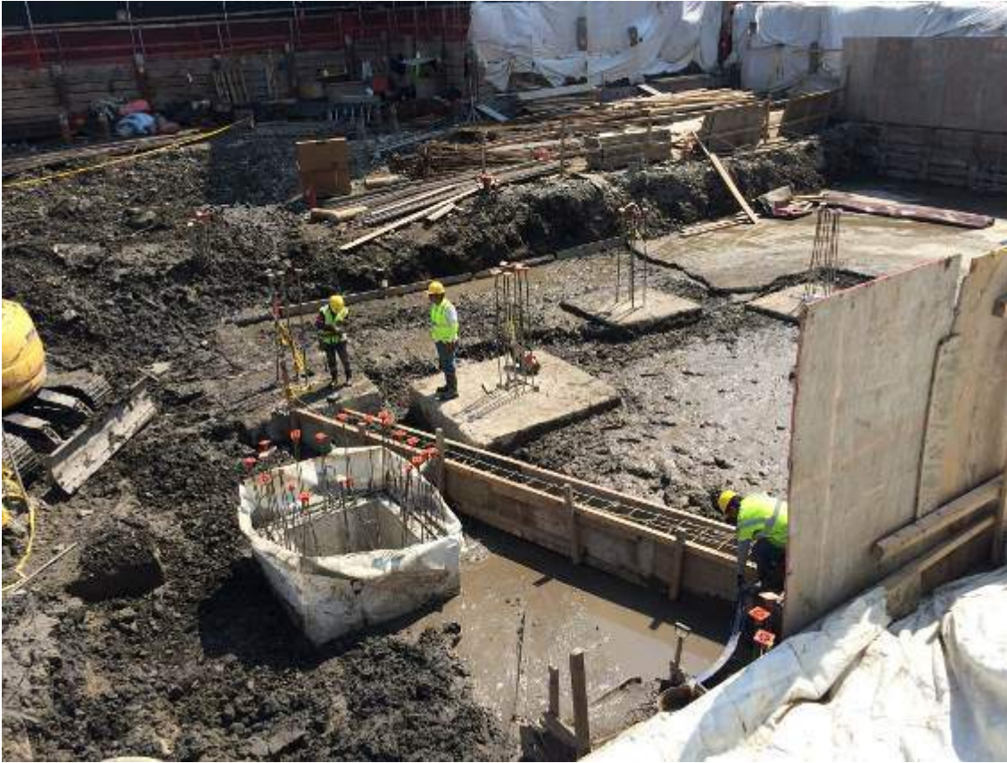
Photograph 57: View of the installed grade beams and sewage ejector pit in the eastern portion of the Site, facing east.
