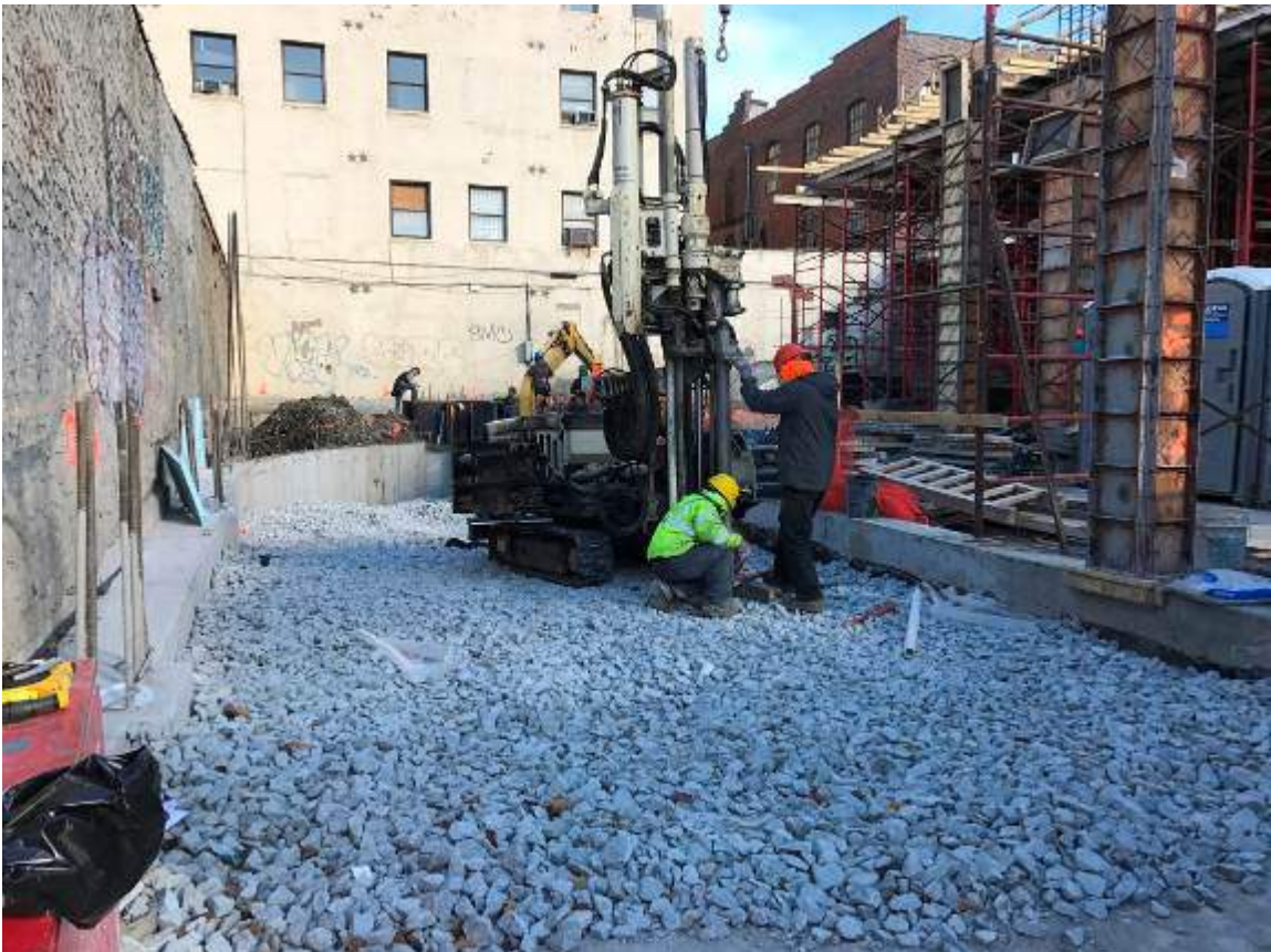
Photograph 124: View of AARCO installing the permanent monitoring well (SMW-2) in the ramp entrance area, facing northeast.
