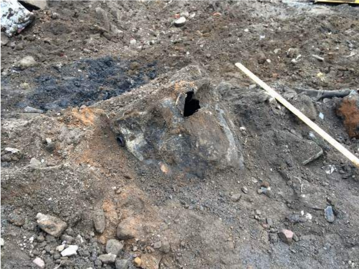
Photograph 11: View of UST-14 discovered in the western portion of the Site.
