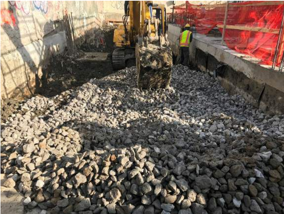
Photograph 123: View of the imported stone being placed in the southern portion of the western ramp, facing north.
