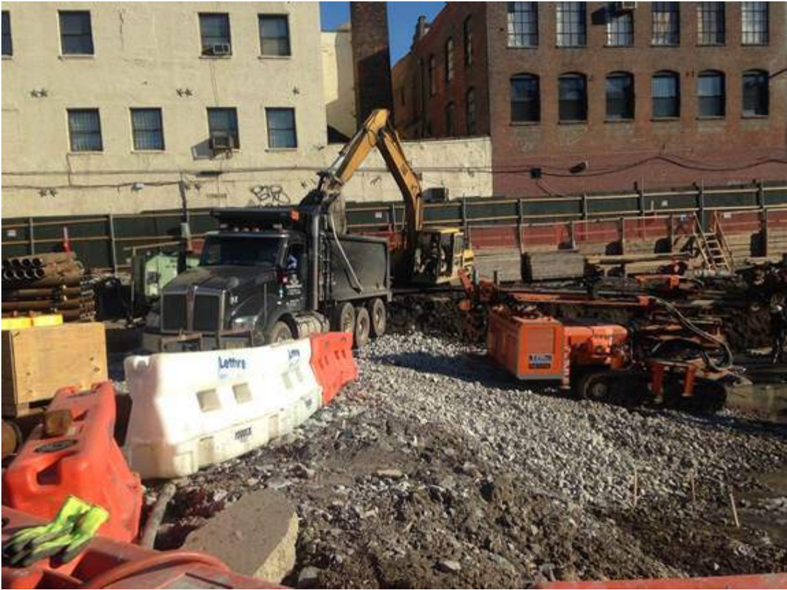
Photograph 49: View of the contractor directly loading material for off-site disposal, facing northeast.
