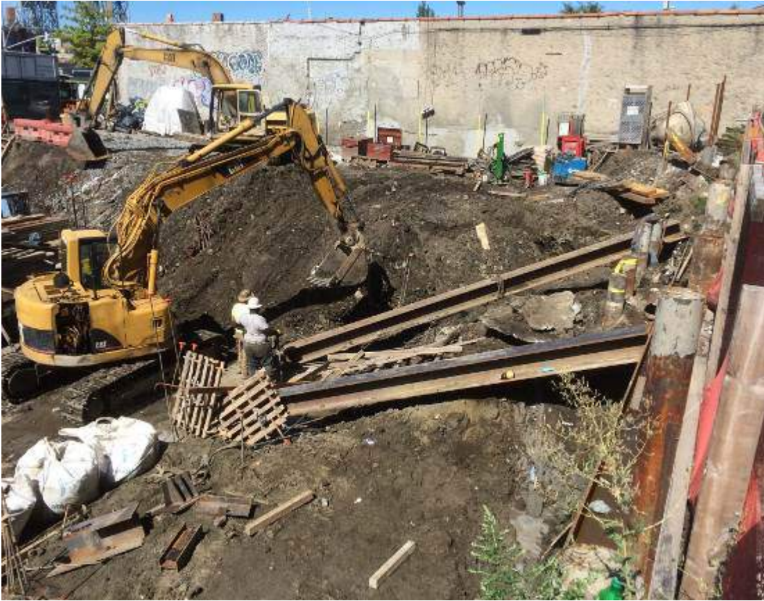
Photograph 85: View of the raker installation along the northwest Site boundary, facing west.
