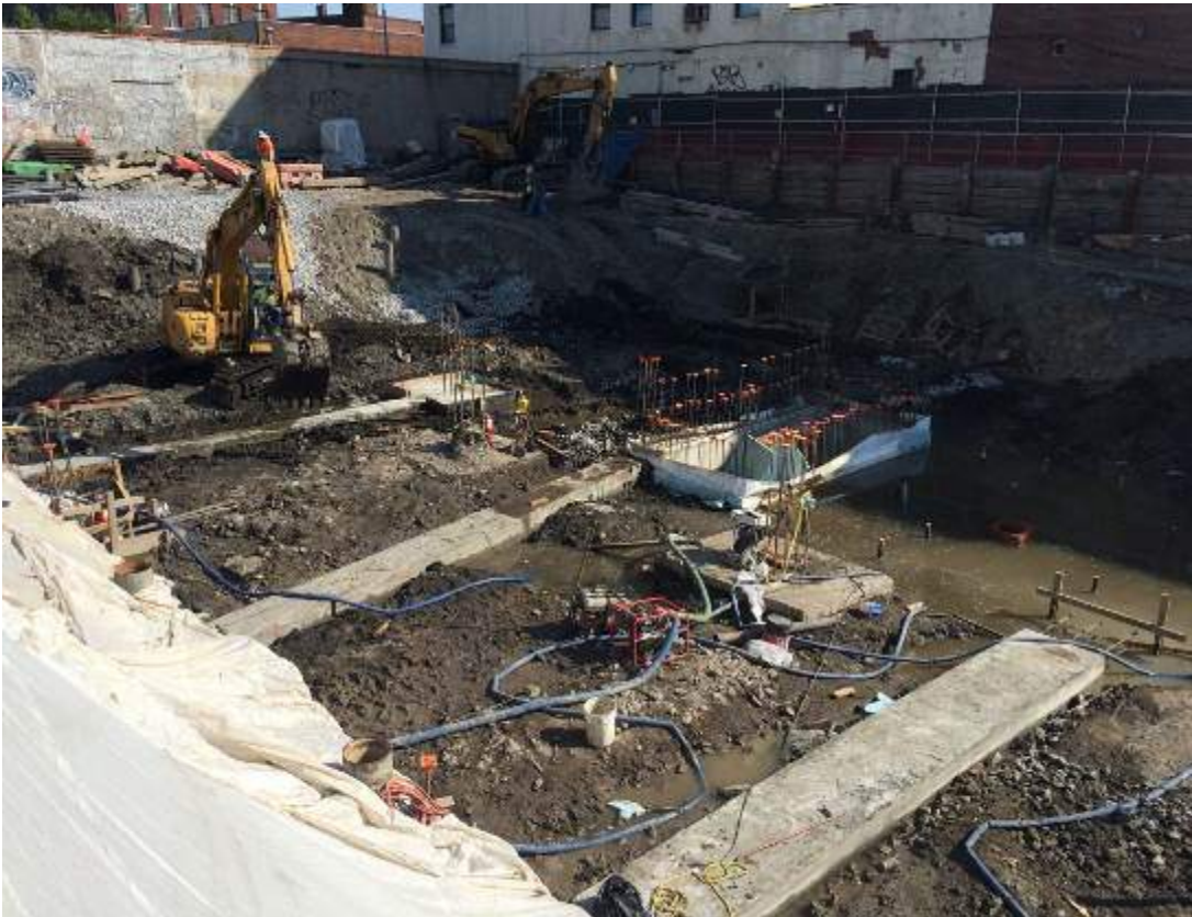
Photograph 60: View of the installed grade beams in the central portion of the Site, facing north.
