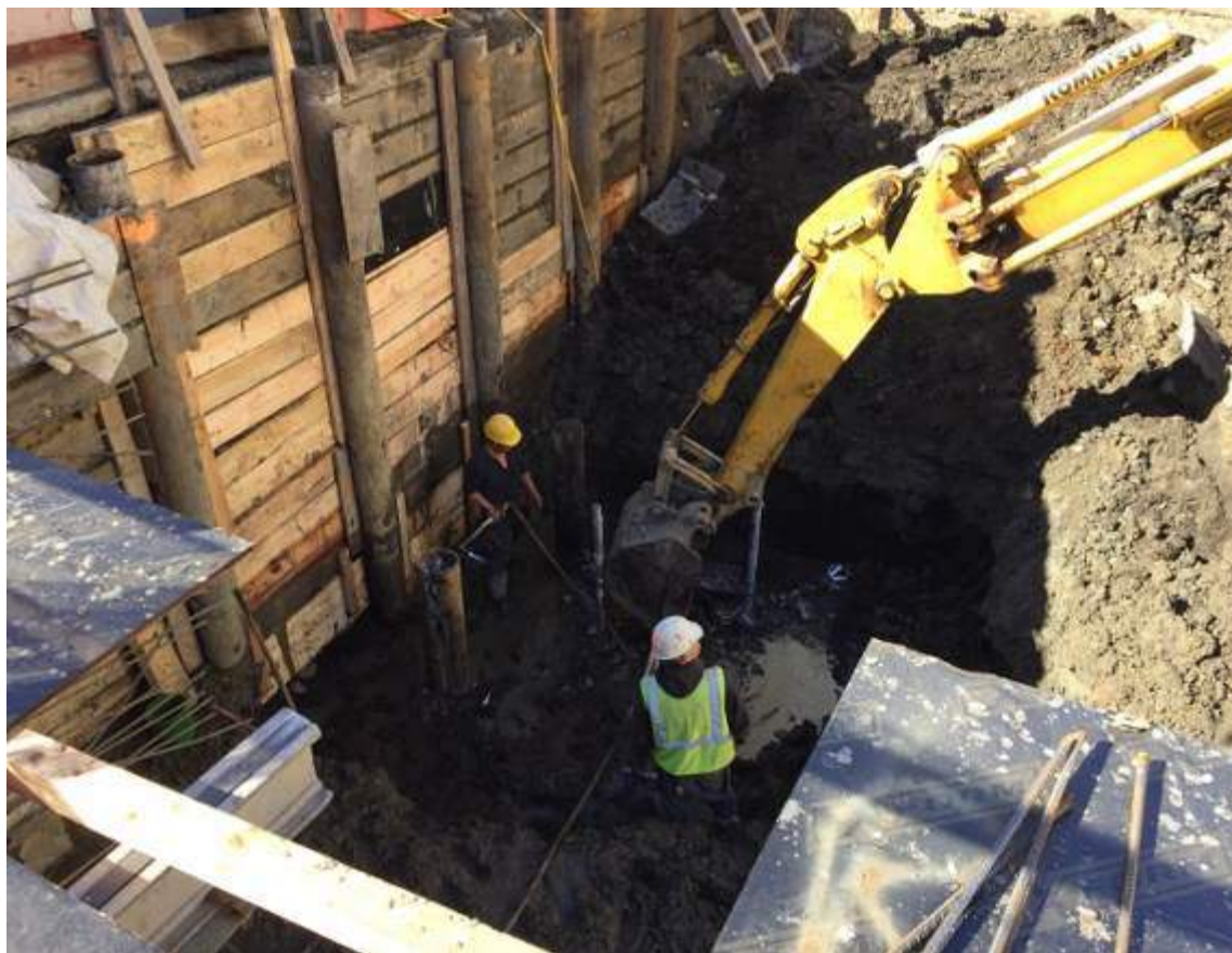
Photograph 116: View of the contractor excavating for a pile cap along the southwestern portion of the site, facing west.
