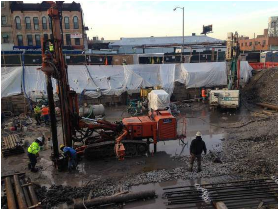
Photograph 51: View of the contractor drilling piles in the central and western portions of the Site, facing west.
