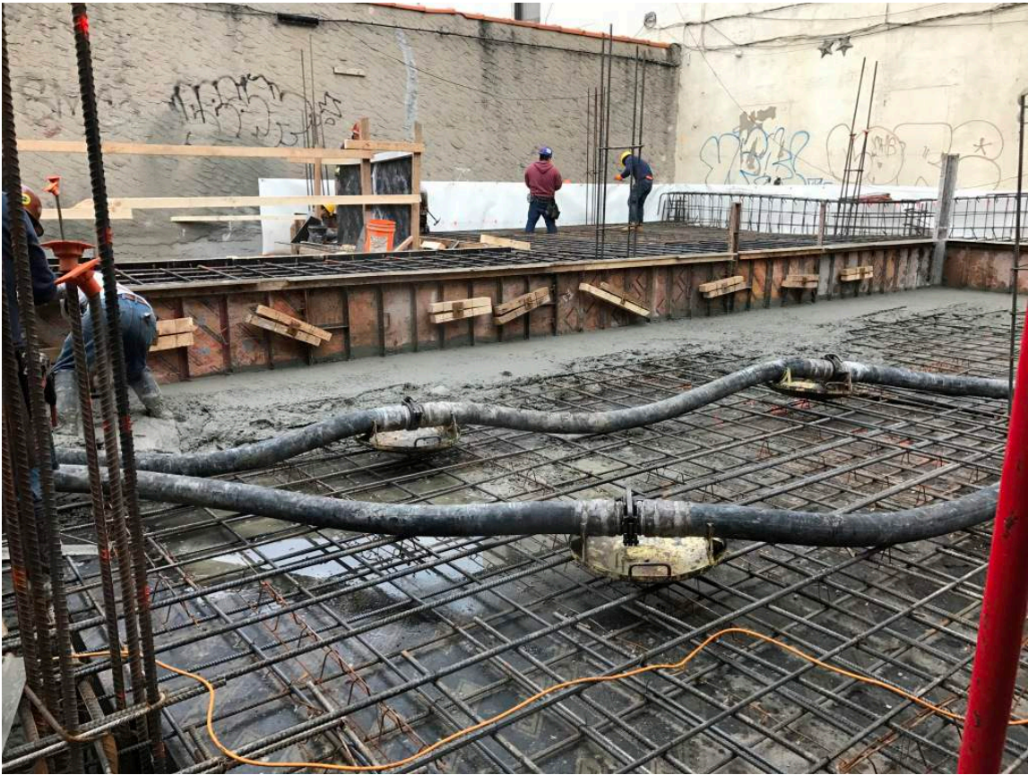
Photograph 133: View of the concrete installation in the northern portion of the Site, facing north.
