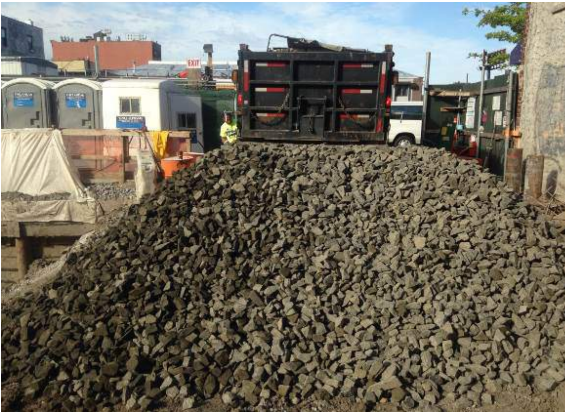
Photograph 76: View of the 3 to 5-inch virgin quarry stone that was delivered to the Site.
