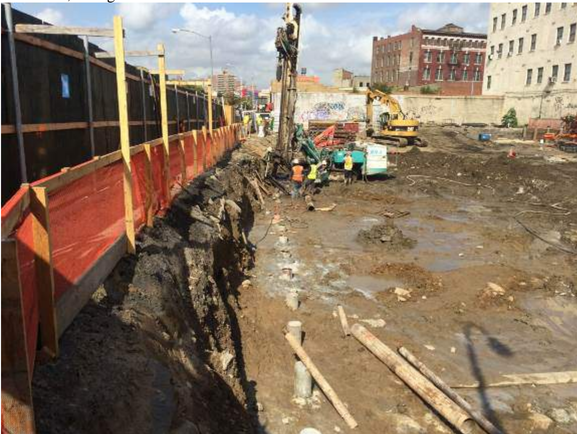
Photograph 28: View of the pile installation along the E. 138 th Street boundary of the Site.
