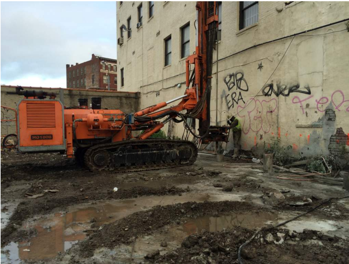
Photograph 3: View of the subcontractor injecting grout into the soil along the northern boundary of the Site, facing north.
