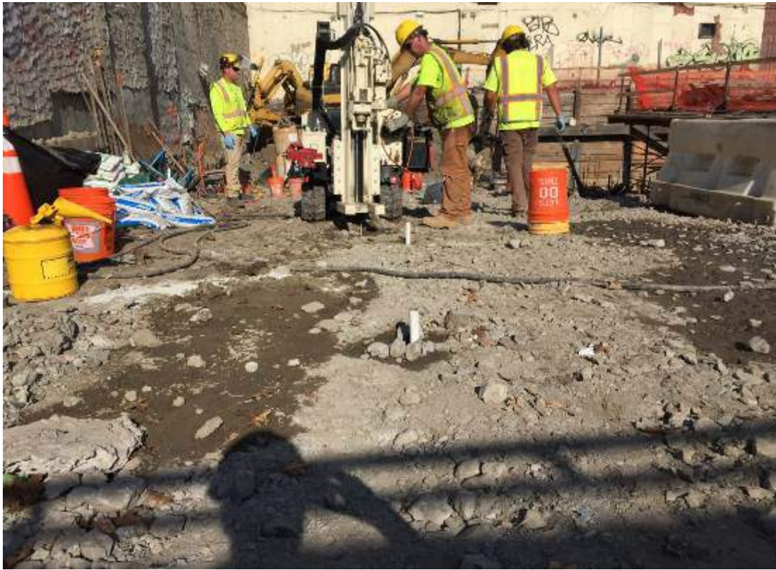
Photograph 97: View of ERFs advancing several one-inch temporary injection well points to gravity feed the reagents into the subsurface, facing northeast.
