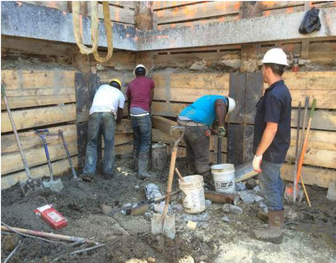
Photograph 81: View of the contractor installing lagging in the northeastern portion of the Site, facing northeast.
