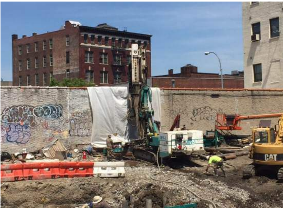
Photograph 54: View of the contractor drilling piles along the western boundary of the Site, facing northwest.
