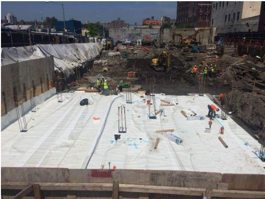
Photograph 58: View of the installed waterproofing membrane in the eastern portion of the site, facing northwest.
