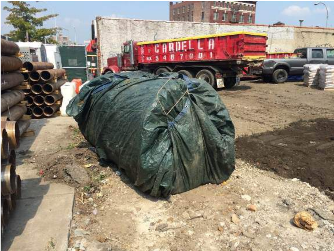
Photograph 15: View of UST-15 removed and covered in plastic along the E. 138 th Street boundary.
