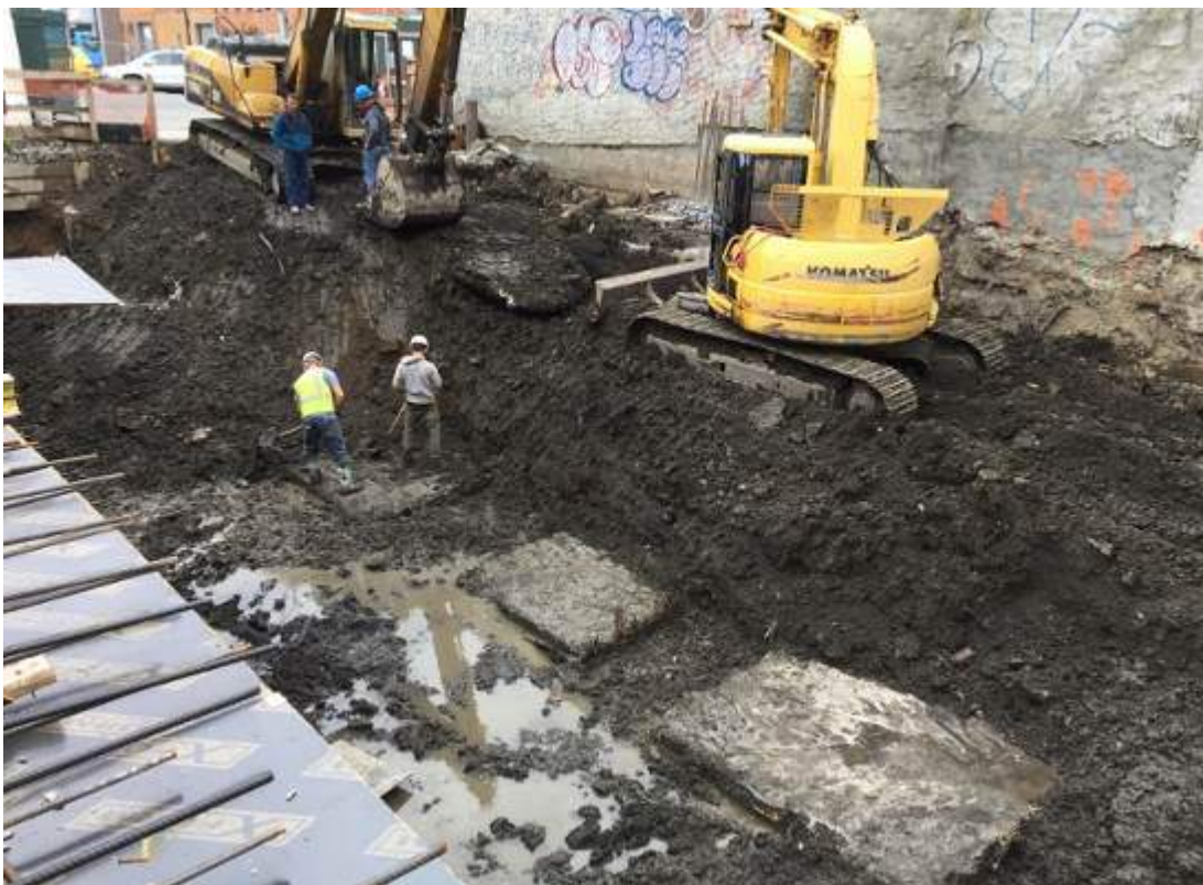
Photograph 110: View of the contractor excavating along the western portion of the site, facing west.
