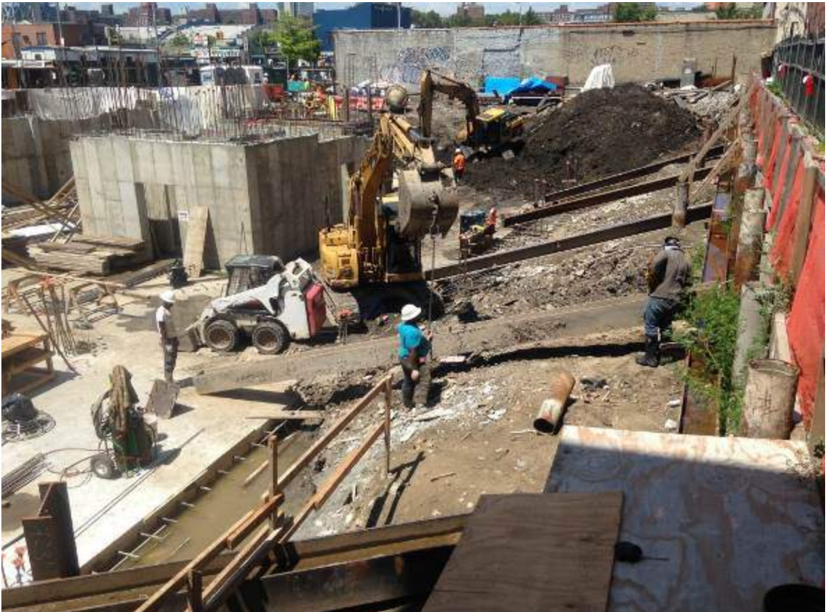
Photograph 70: View of the contractor installing rakers along the northern boundary of the site, facing northwest.
