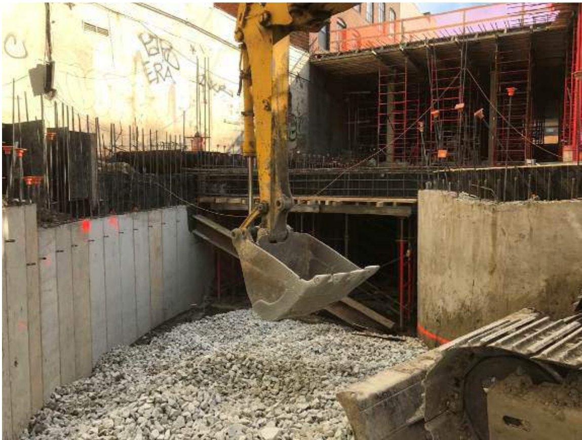
Photograph 125: View of the northern portion of the ramp descending into the basement, facing east.
