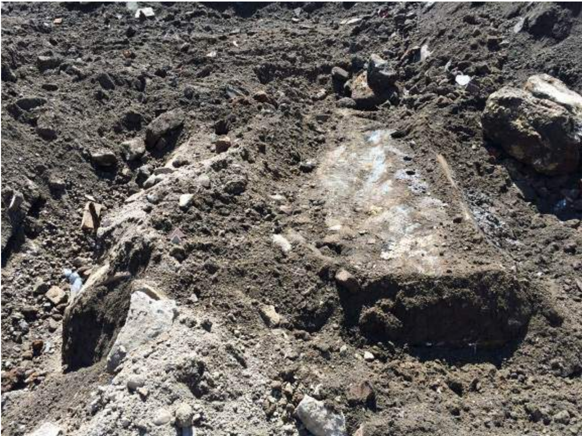
Photograph 6: View of the two (2) USTs (UST-12 and UST-13) encountered during excavation in the southern portion of the Site.
