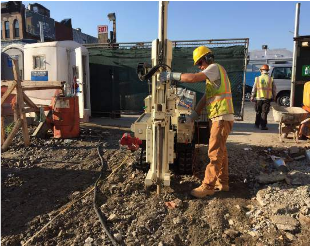
Photograph 93: View of ERFS installing the on-site temporary monitoring well (TMW-2), facing southwest.
